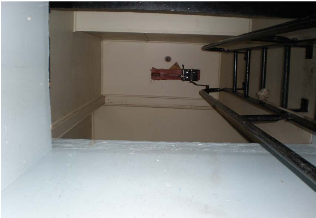
Photo 16/4 - Bonded asbestos lining in plant room (above Room 23)
