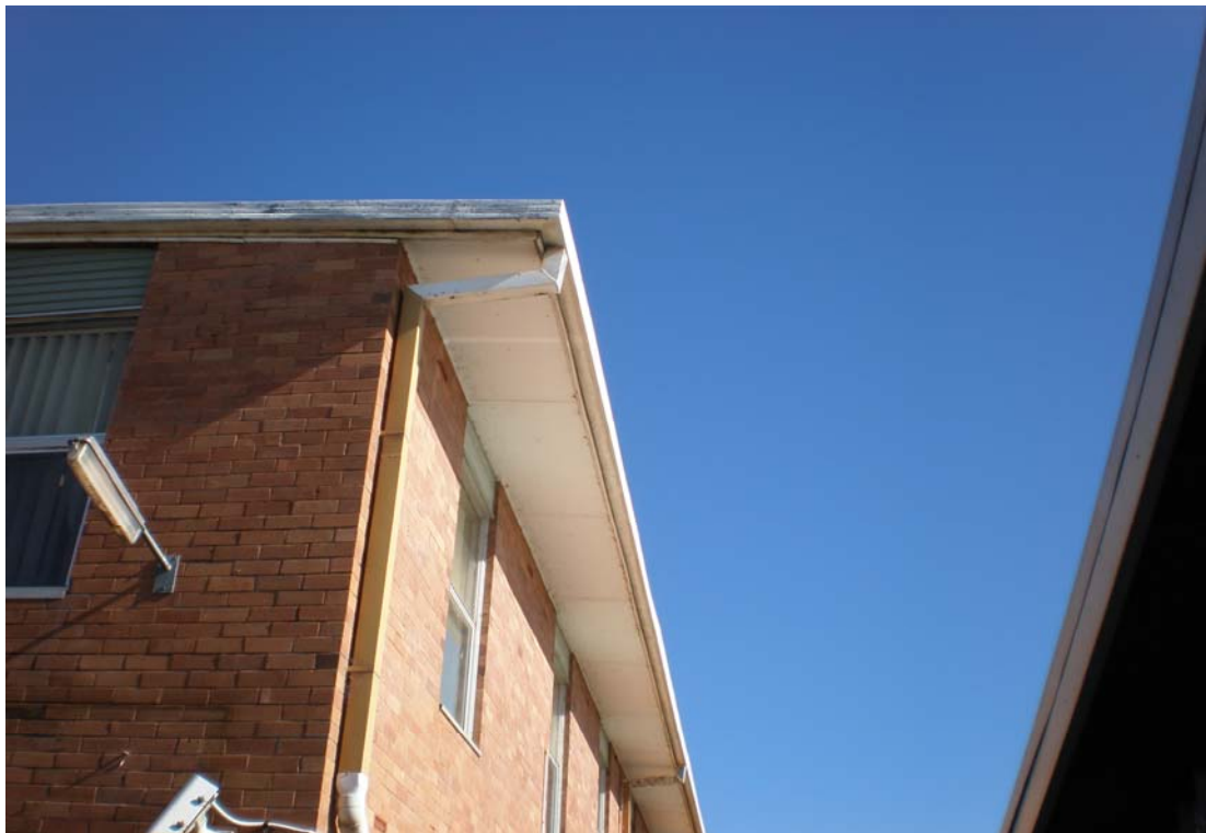
Photo 16/2 - Bonded asbestos eve lining
