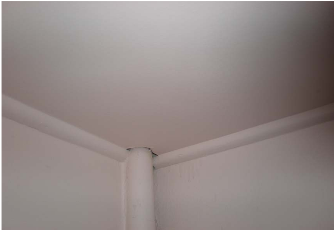
Photo 16/7 - Bonded asbestos ceiling in fire hose cupboard #2
