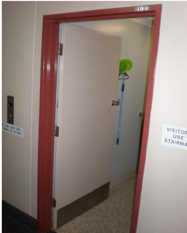
Photo 16/3 - Fire door (Room 23) with friable asbestos core
