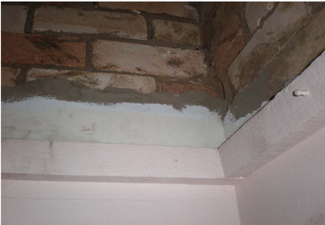
Photo 16/6 - Potential asbestos lining above former asbestos ceiling in fire hose cupboard #1
