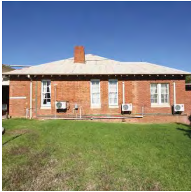
Figure 92 c1890/1926 additions exterior north face showing modifications to wall including the junction between the two
