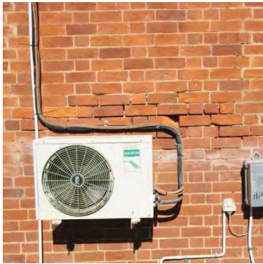
Figure 95 c1890 external wall where the soft bricks are being seriously damaged by air conditioning unit – the units need to be removed
