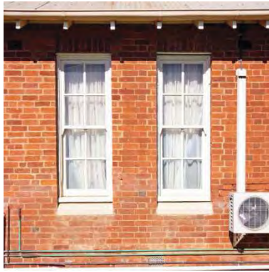
Figure 93 c1890 additions exterior north face showing 1926 windows cut into wall. The discoloured mortar shows where bricks were removed.
