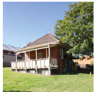
Figure 100 1936 kiosk – from south west. This building is largely intact but could be presented better
