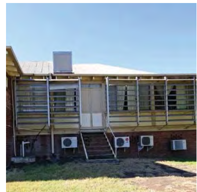
Figure 91 1926 additions to 1868 building exterior showing verandah. The c1970 louvres have not survived well and are now detracting from the building
