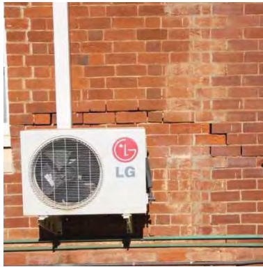
Figure 96 c1890 external wall at junction with 1926 addition where the stronger bricks are not suffering as greatly.
