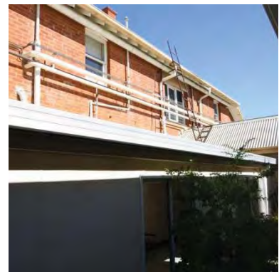
Figure 73 1907 building exterior rear showing how hospital services can impact heritage. Generally there is sensitivity in the servicing of the old building.
