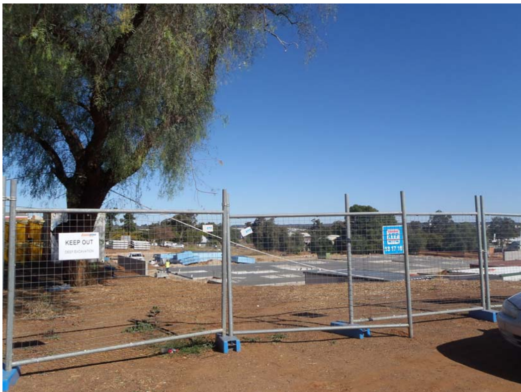
Plate 3: view south west across new construction area to the western section (note this construction was started before survey)
