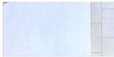
D – WHITE PAINTED CONCRETE CANDALEPAS ASSOCIATES – PINDARI
