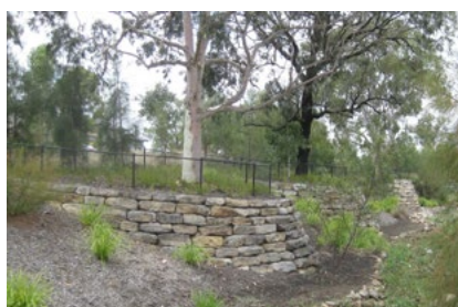
Figure 50-49: An example of fencing around a rock battered drainage channel.
