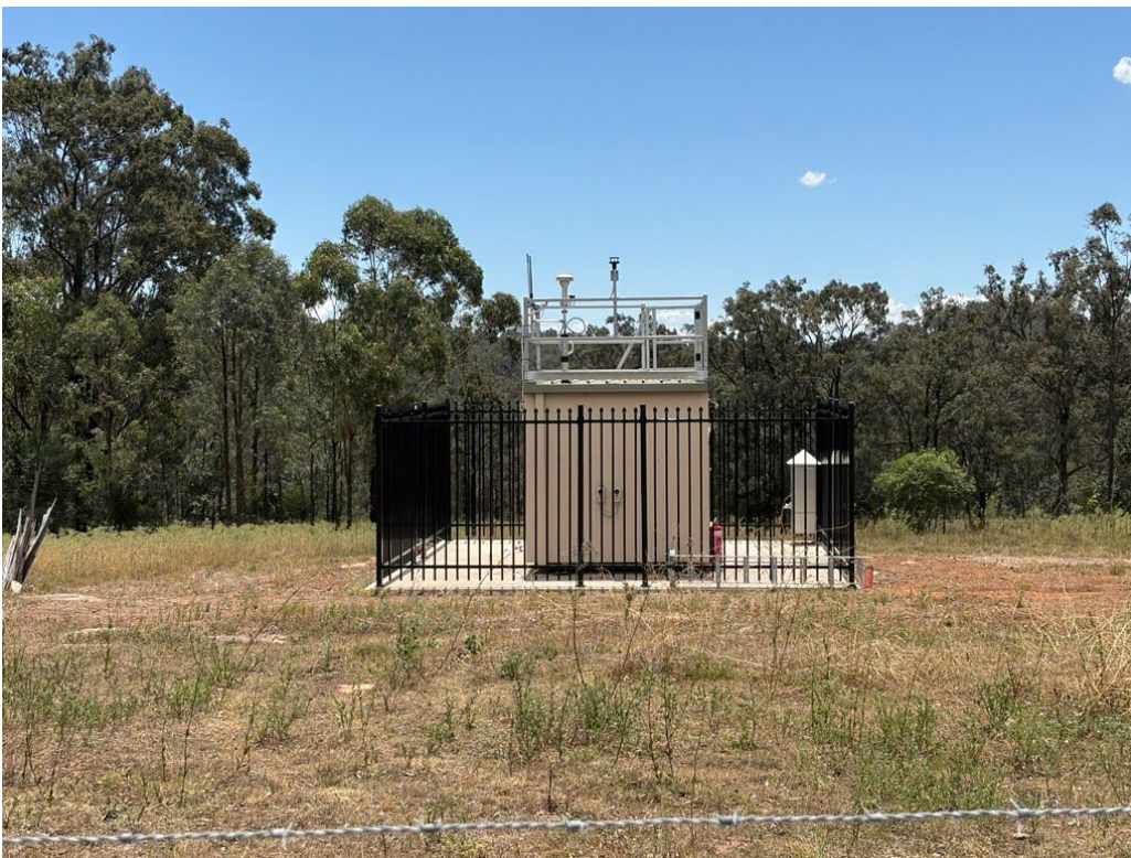
Plate 8: Roxburgh Road TEOM, noting substandard installation of the depositional dust gauge against fence (Inspection date 26/11/2025).
