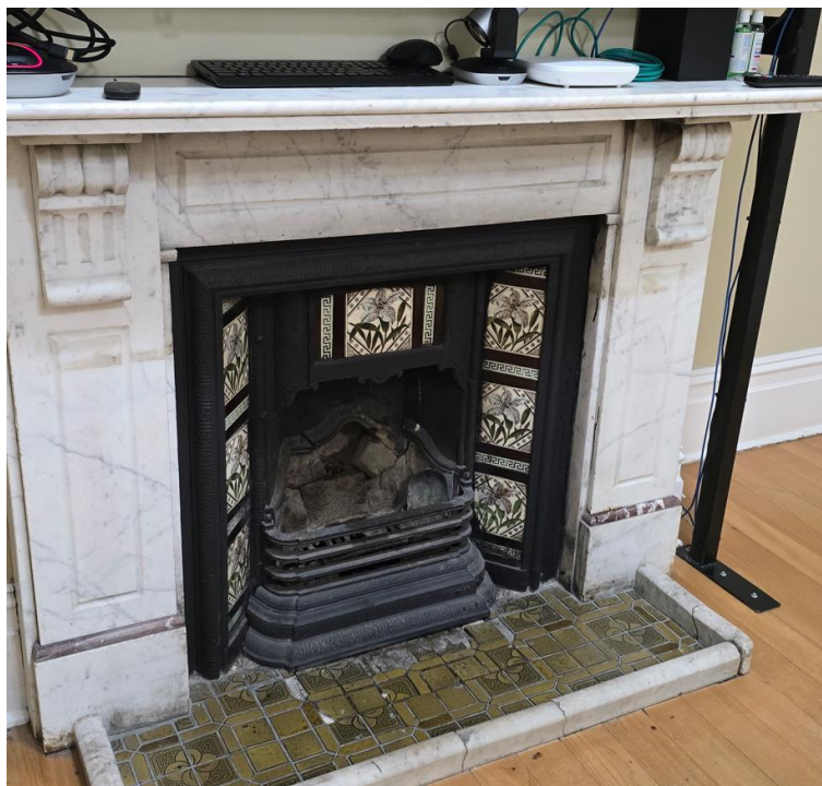
Internal views of fire places
