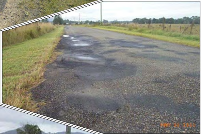
Plate 4.2: Waukivory Road - example of pavement failure. (Ref: Constructive Solutions 2016 - Plate 2)
