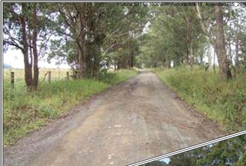
Plate 4.5: McKinleys Lane - typical alignment and condition. (Ref: Constructive Solutions 2016 - Plate 7)
