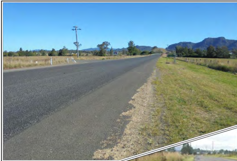
Plate 4.1: The Bucketts Way east of Gloucester - typical alignment and condition. (Ref: Constructive Solutions 2016 - Plate 3)
