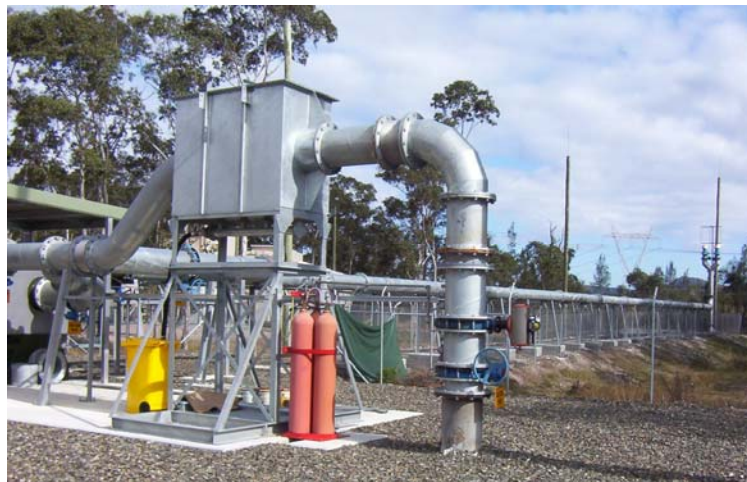
Plate 4 – Methane Gas Drainage Plant at the Mandalong Mine Access Site
