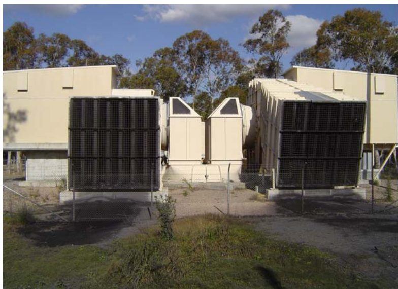
Plate 3 – Ventilation Fans at the Mandalong Mine Access Site
