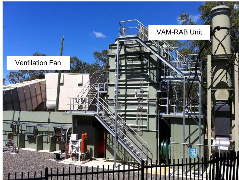
Plate 6 – VAM-RAB Trial Unit at Mandalong Mine Access Site
