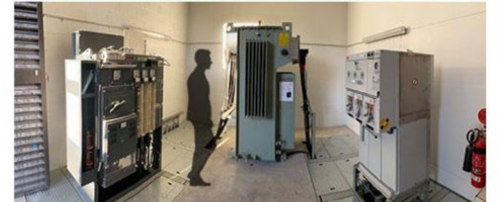
Inside a chamber substation
