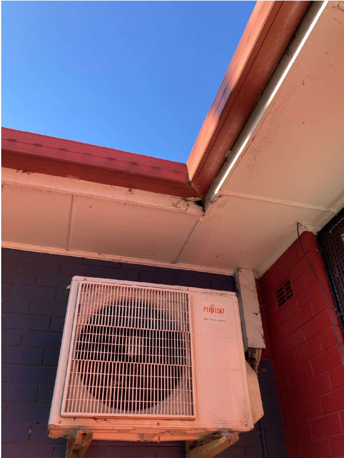
Figure 22: One of the gaps in awning of roof of the PCYC building that was not surveyed with an ultrasonic detector
