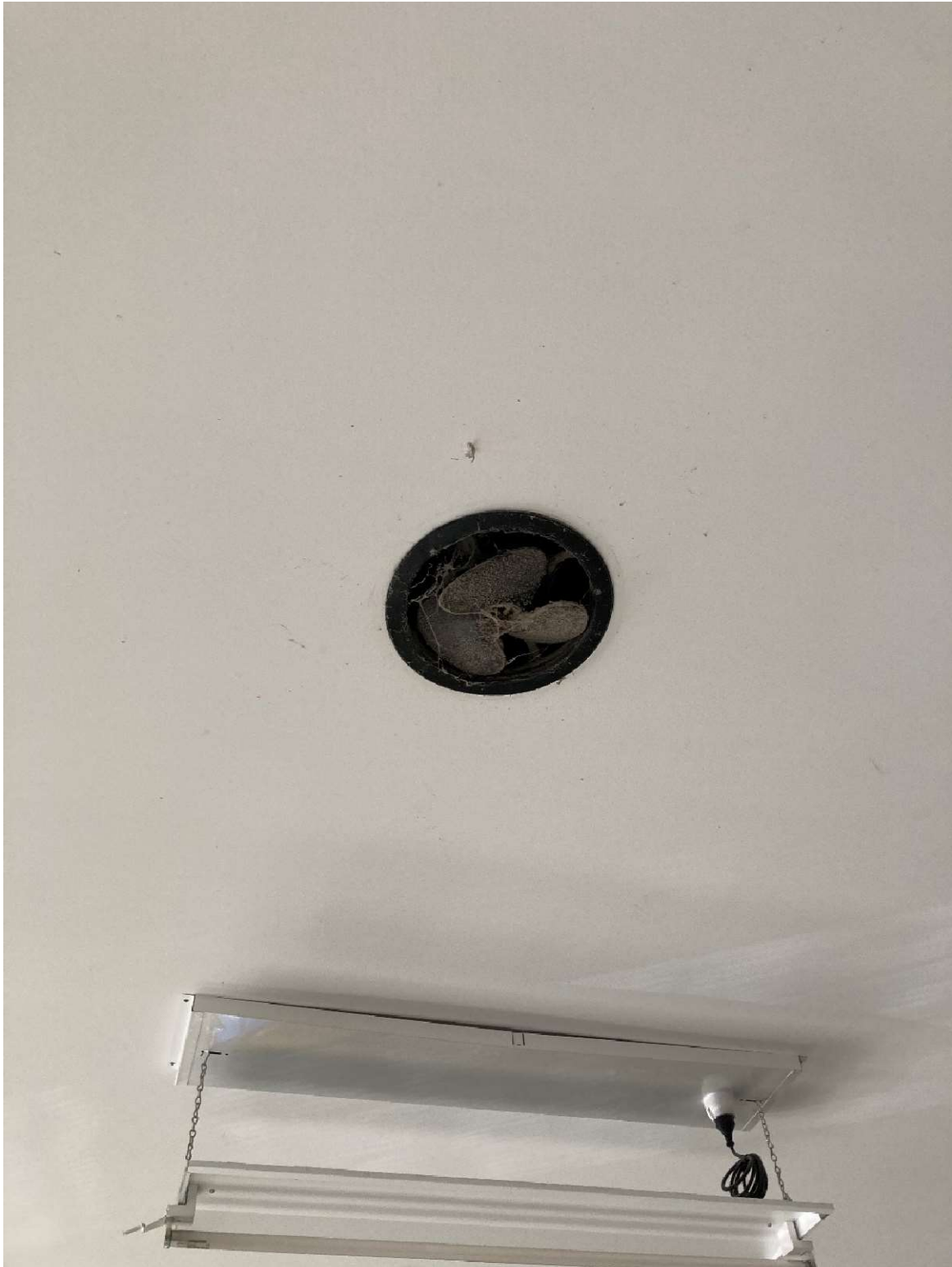
Figure 18: An opening the ceiling. The Anabat SD2 ultrasonic detector was directed at the opening to listen for microbat vocalisations.
