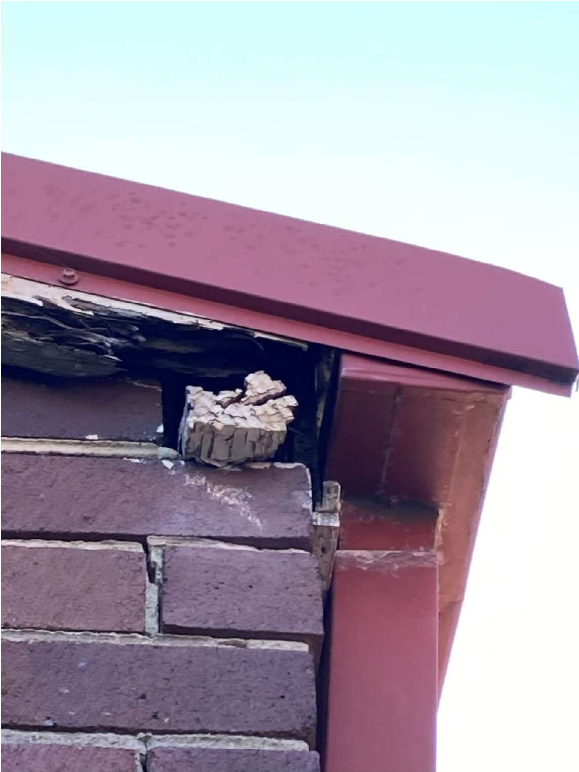
Figure 21: One of the gaps in awning of roof of the PCYC building that was surveyed with an ultrasonic detector
