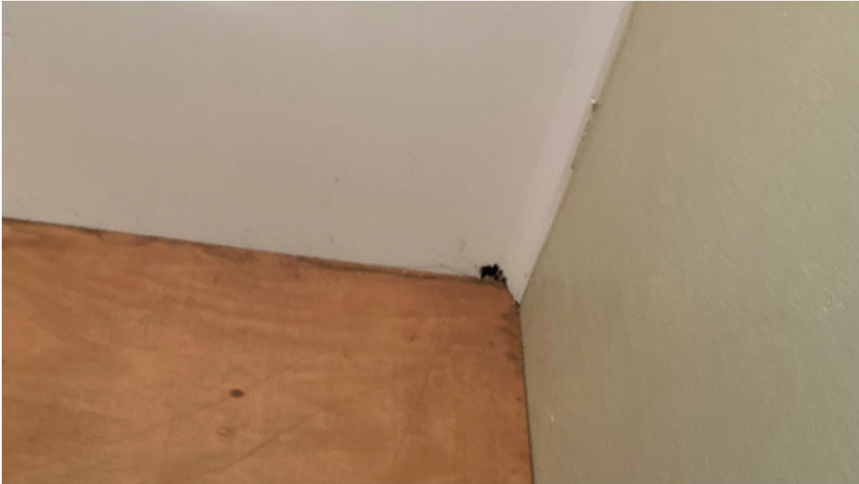
Figure 19: An opening in the corner of the room. The Anabat SD2 ultrasonic detector was directed at the opening to listen for microbat vocalisations.
