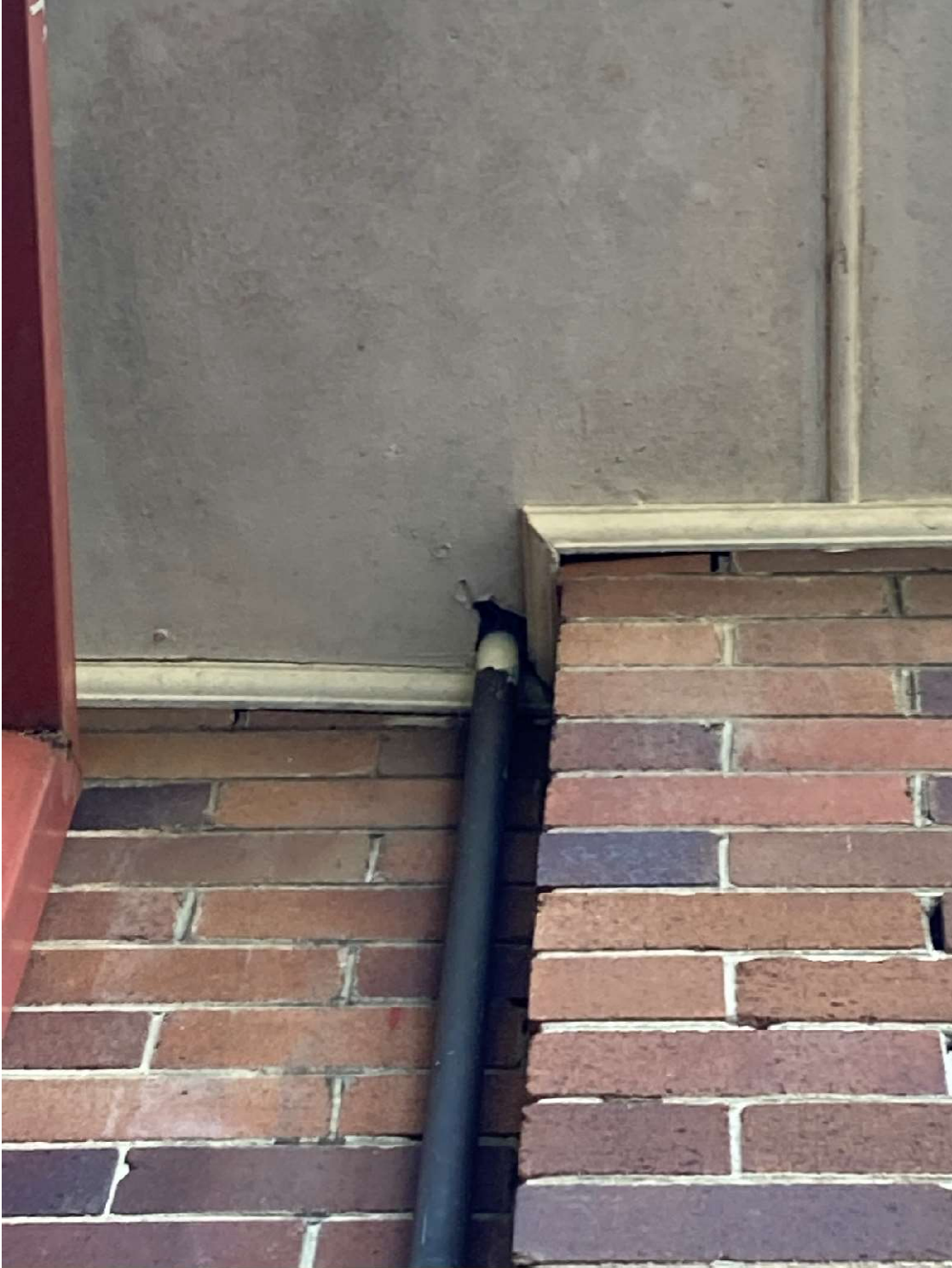
Figure 23: One of the gaps in awning of roof of the PCYC building that was not surveyed with an ultrasonic detector
