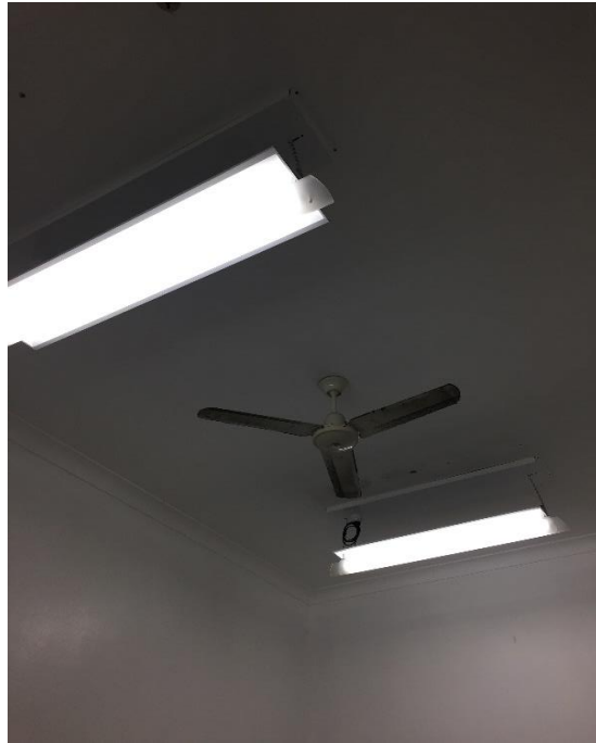
Photograph 29: PCYC, interior, storage 6, ceiling, fan x 1, capacitors, insulating oil, PCB (assumed)
