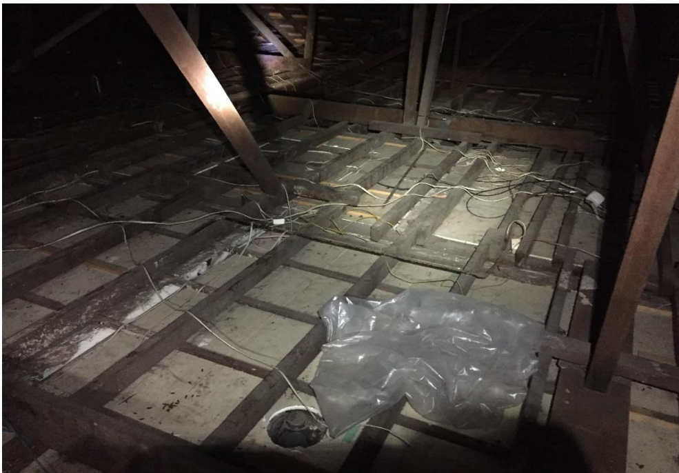
Photograph 32: PCYC, interior, ceiling cavity, northern end of building (near storage 4), settled dust/debris, 280 mg/m2 lead
