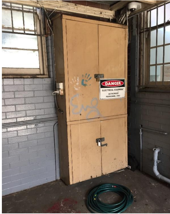
Photograph 3: PCYC, exterior, covered courtyard at centre of building, electrical cabinet, internal components, electrical backing board, fuse insulation and/or other materials, asbestos (assumed)
