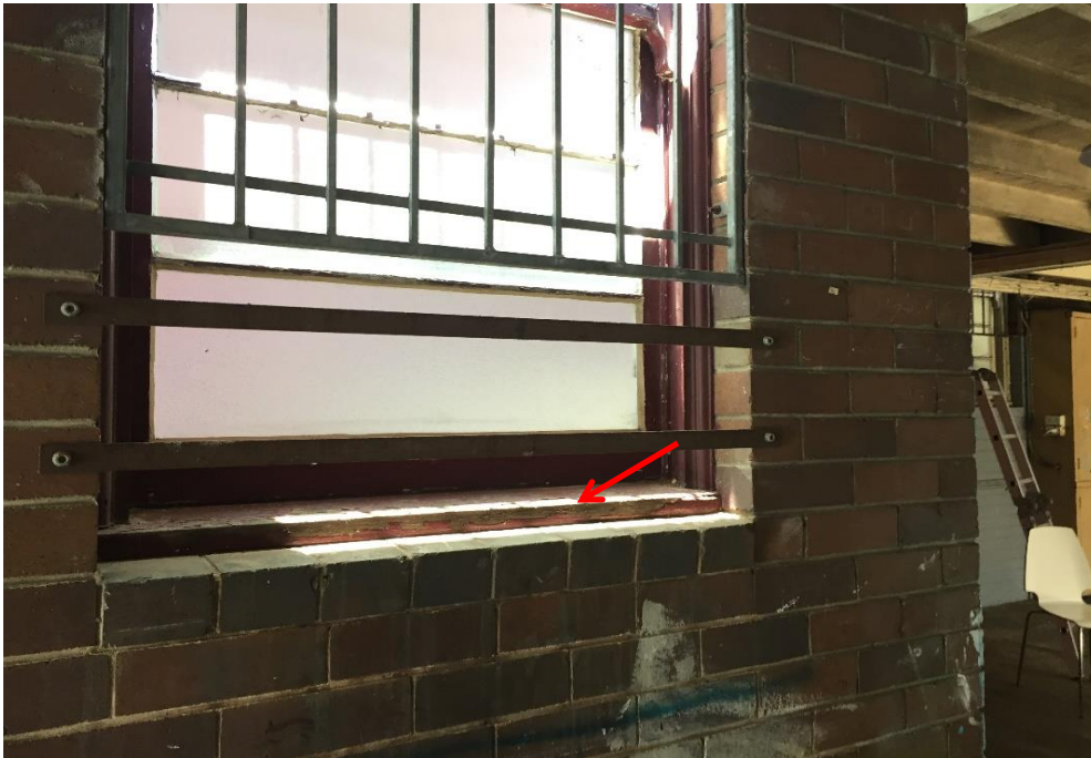
Photograph 21: PCYC, exterior, covered courtyard at centre of building, southern side, timber window frame, typical burgundy paint, lead paint (>0.1% lead w/w)
