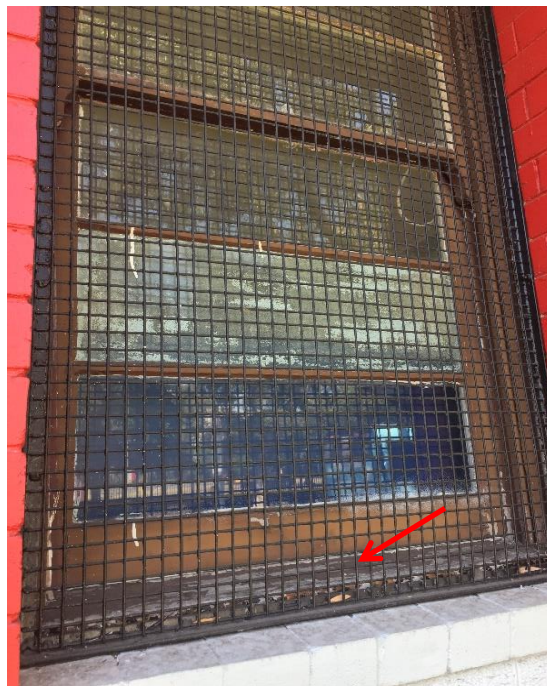
Photograph 18: PCYC, exterior, western façade, north end building, typical window frame, brown paint, lead paint (>0.1% lead w/w)
