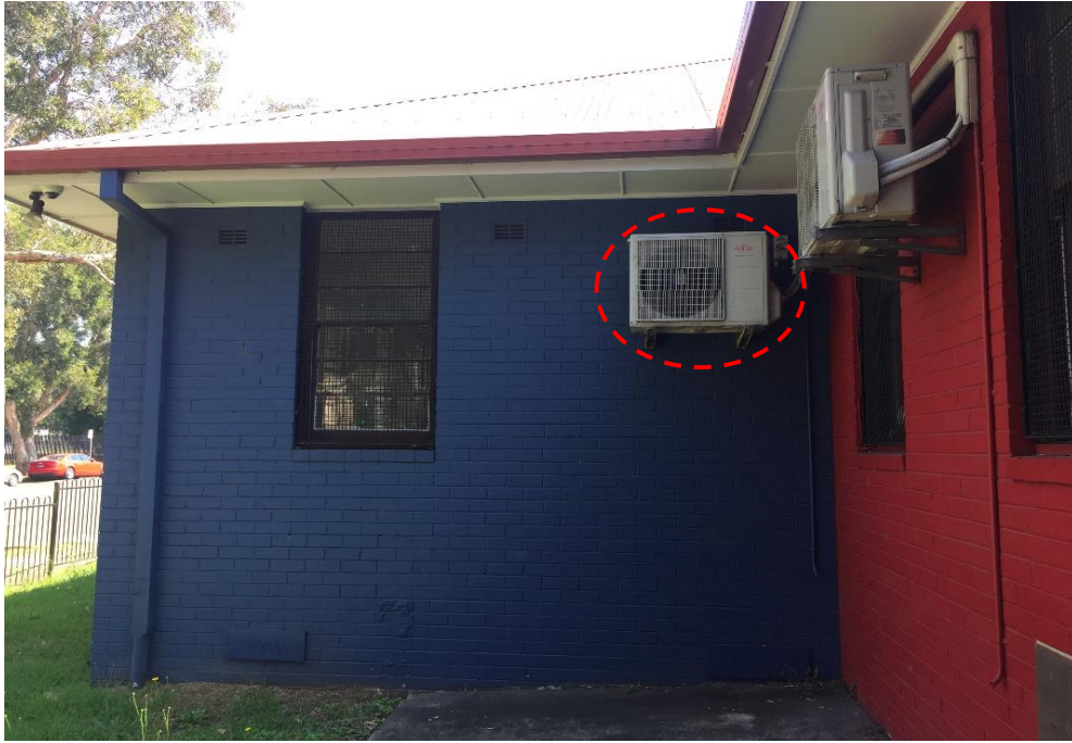
Photograph 23: PCYC, exterior, western façade, adjacent north of main entrance, Fujitsu AC unit, refrigerant, refrigerant R32
