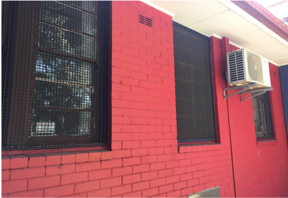
Photograph 25: PCYC, exterior, western façade, adjacent south of main entrance, AC unit, refrigerant, refrigerant R32
