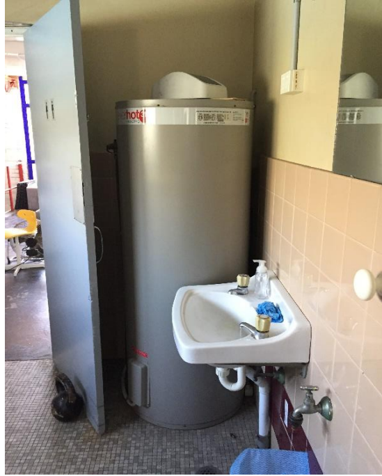
Photograph 31: PCYC, interior, mezzanine off weight gym 2, amenities area, hot water unit, insulation, SMF (assumed)
