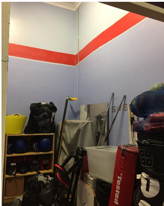
Photograph 12: PCYC, interior, stationary store, portion of wall linings, fibre cement sheeting, asbestos detected by analysis
