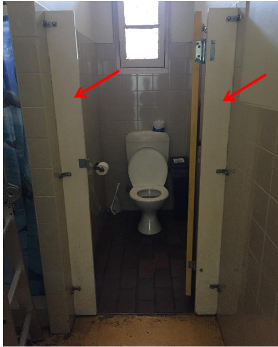
Photograph 13: PCYC, interior, police changing room, partitions, possible fibre cement product, asbestos (assumed)
