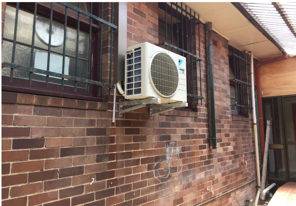
Photograph 26: PCYC, exterior, central passageway / courtyard, Daikin AC unit, refrigerant, refrigerant R32
