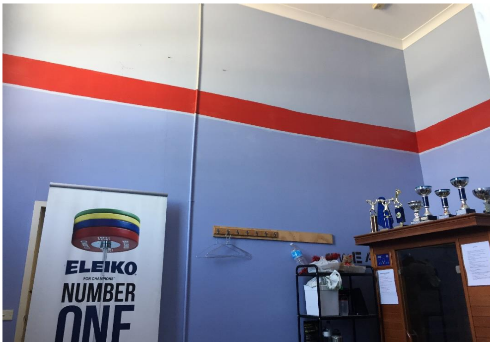
Photograph 8: PCYC, interior, storage 7, portion wall linings, fibre cement sheeting, asbestos detected by analysis
