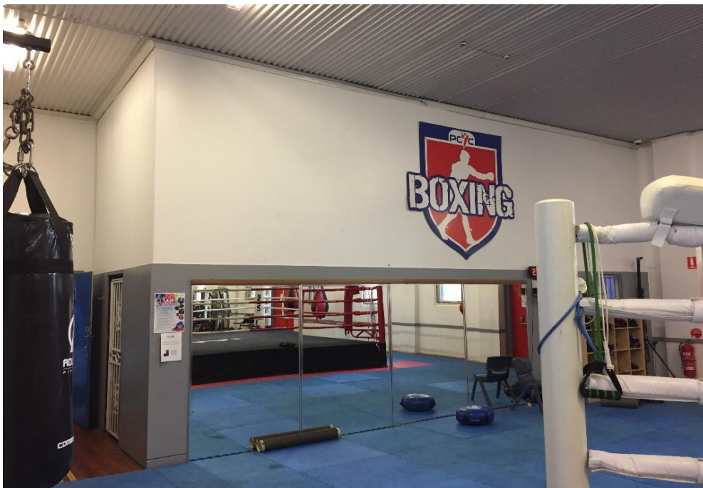
Photograph 10: PCYC, interior, gym/boxing, eastern wall (adjacent storage 7 and stationary store), fibre cement sheeting, asbestos detected by analysis
