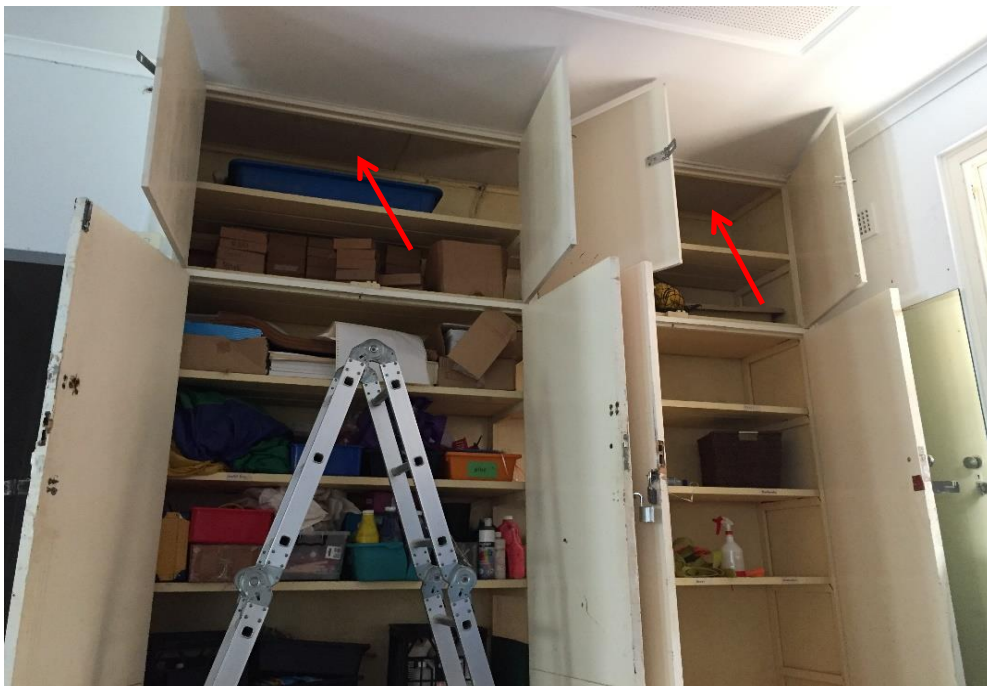
Photograph 4: PCYC, interior, dance studio, southwestern corner, cupboards, ceiling lining, fibre cement sheeting, asbestos (assumed)
