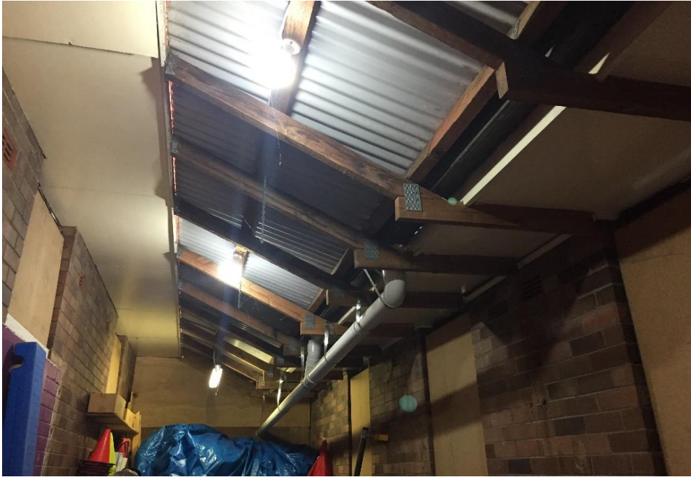
Photograph 5: PCYC, interior, photo room, continuation of eave linings throughout, fibre cement sheeting, asbestos (assumed)
