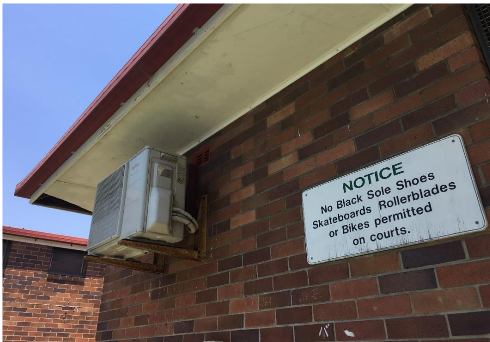
Photograph 22: PCYC, exterior, eastern façade, eastern side of dance studio, Fujitsu AC unit, refrigerant, refrigerant R32
