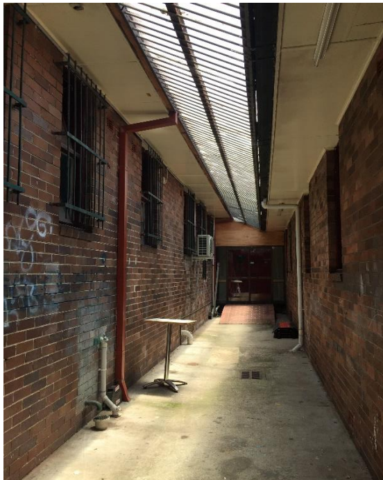
Photograph 2: PCYC, exterior, central passageway, dance studio, western eave lining, fibre cement sheeting, asbestos detected by analysis
