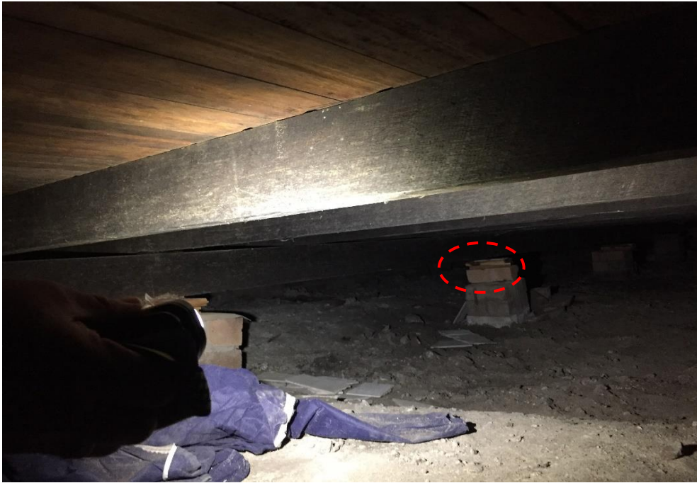
Photograph 17: PCYC, exterior, below dance studio, subfloor area, packing materials to brick piers, fibre cement sheeting, asbestos (assumed)
