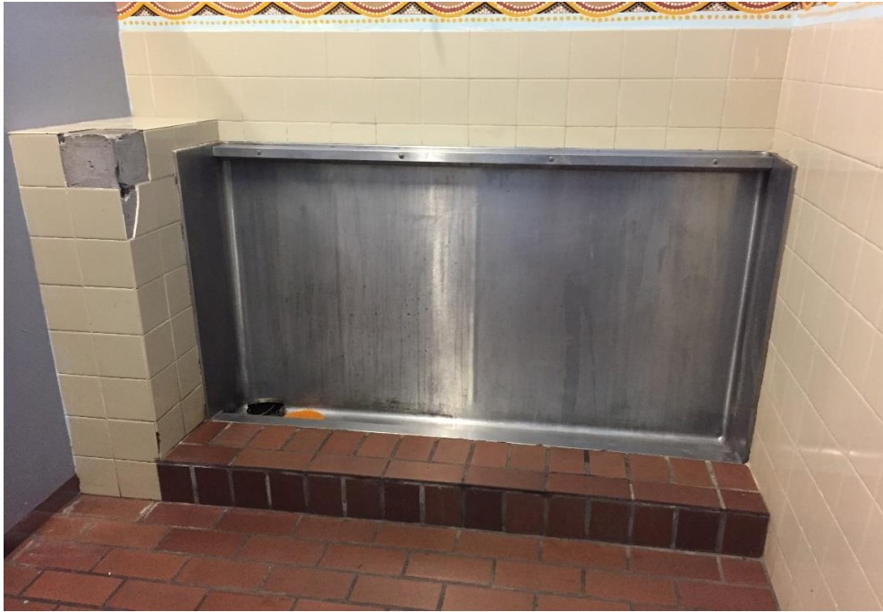
Photograph 7: PCYC, interior, male toilets (adjacent north of police change room), rear side of urinal, possible bituminous lining/coating, asbestos (assumed)
