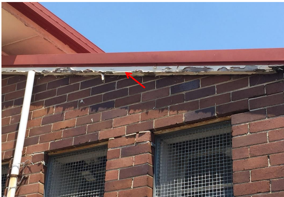
Photograph 20: PCYC, exterior, eastern façade, southern end of building, fascia, typical cream paint, lead paint (>0.1% lead w/w)
