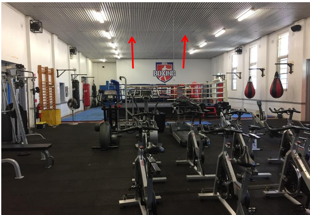
Photograph 30: PCYC, interior, gym/boxing, above perforated metal sheeting to ceiling, insulation, SMF (assumed)
