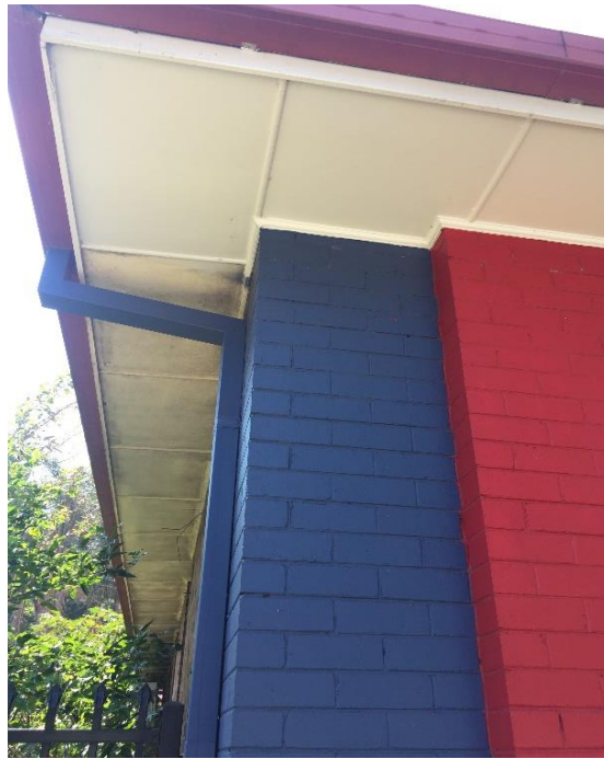
Photograph 1: PCYC, exterior, western façade, northern end, eave lining, fibre cement sheeting, asbestos detected by analysis
