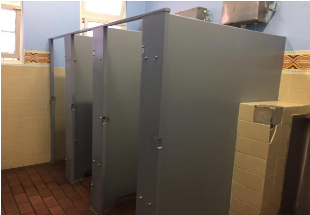
Photograph 6: PCYC, interior, male toilets (adjacent north of police change room), partitions, possible fibre cement product, asbestos (assumed)
