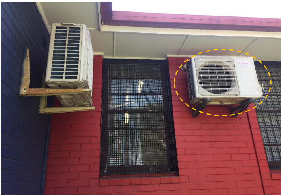
Photograph 24: PCYC, exterior, western façade, adjacent north of main entrance, Fujitsu AC unit, refrigerant, refrigerant 410A
