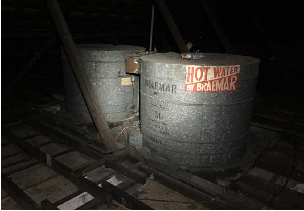
Photograph 15: PCYC, interior, ceiling cavity , hot water tanks (x2) in vicinity of main entrance foyer, internal insulation, asbestos (assumed)
