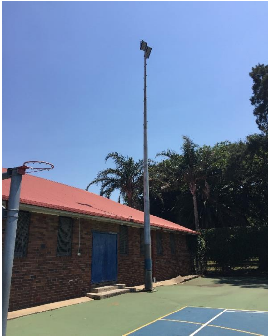
Photograph 27: PCYC, exterior, sports court, light poles, internal components, capacitors (if present), PCB (assumed)
