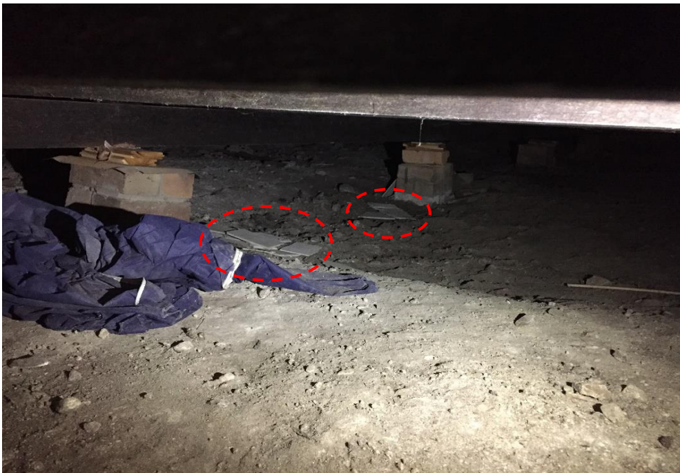
Photograph 16: PCYC, exterior, below dance studio, subfloor area, ground surfaces, fibre cement sheeting debris, asbestos (assumed)
