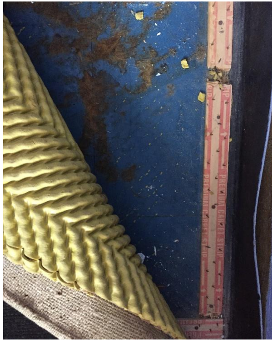
Photograph 9: PCYC, interior, storage 7, floor, below carpet, blue vinyl tiles, asbestos detected by analysis
