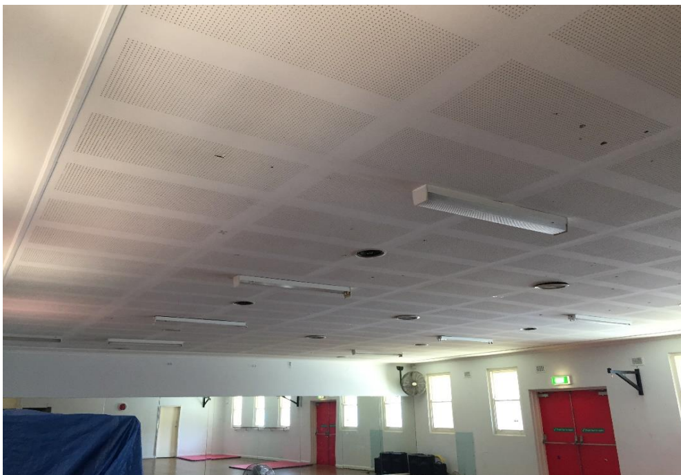
Photograph 28: PCYC, interior, dance studio, ceiling, fluorescent light fittings x 10, capacitors, insulating oil, PCB (assumed)
