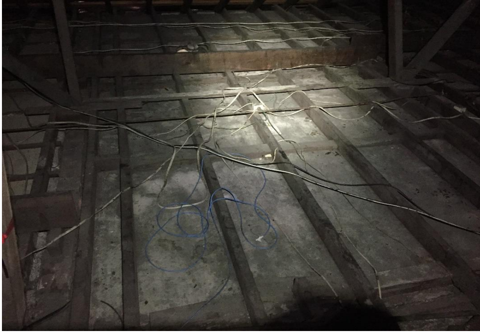
Photograph 33: PCYC, interior, ceiling cavity, toward southern end of building (near office 2), settled dust/debris, 380 mg/m2 lead
