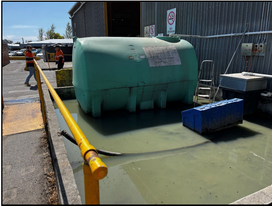
Photo 3: Quarantine wastewater AST and oil/water separator in bund adjacent to the Shed D near the truck wash bay. Looking to the north.
