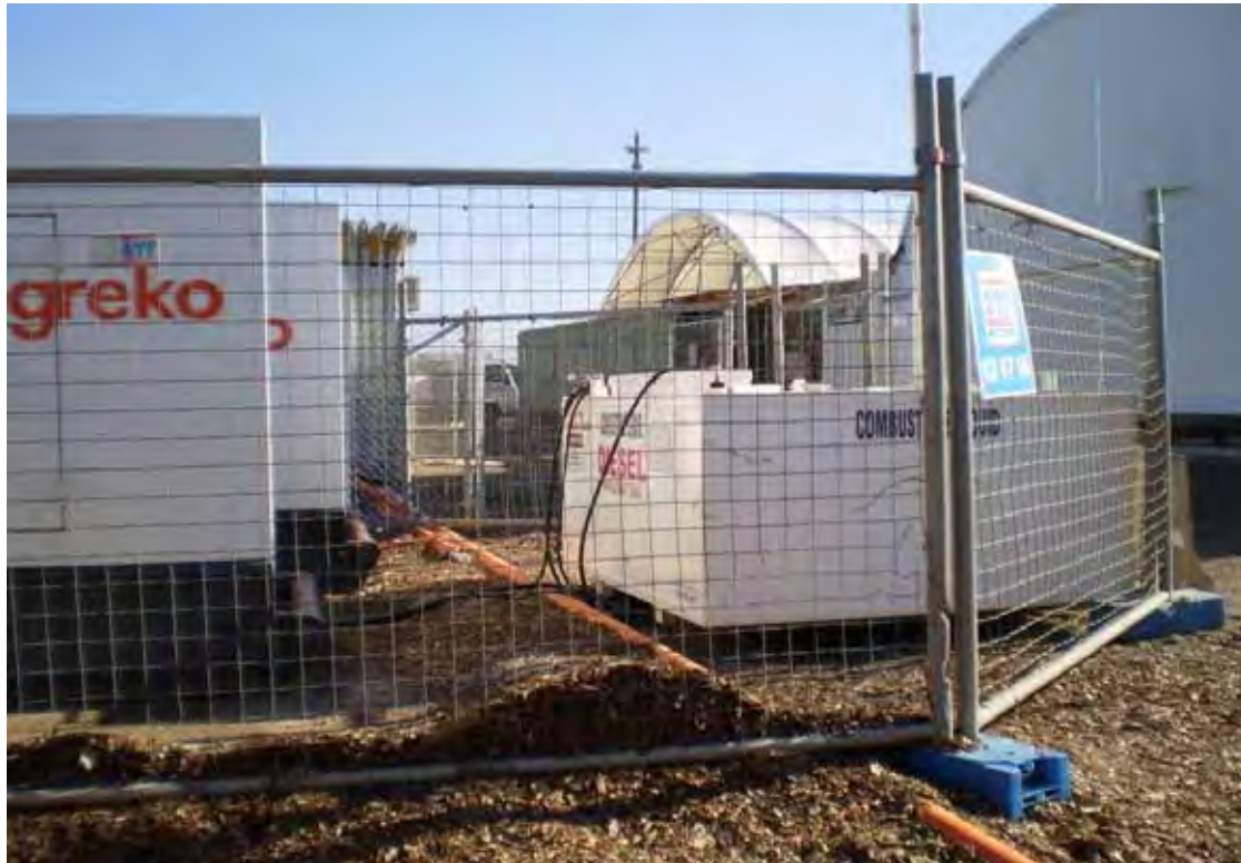
Photo 3 (August 2011) - Generator and diesel tank for refuelling located near site office sheds
