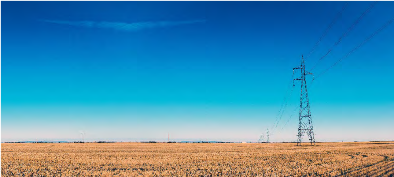
Photograph 3.2 Example of an overhead transmission line
