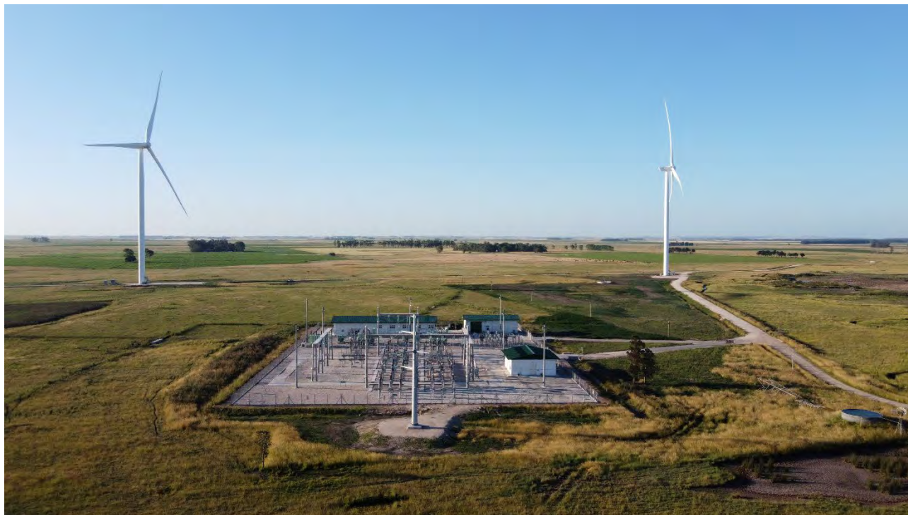
Photograph 3.1 Example of a substation
