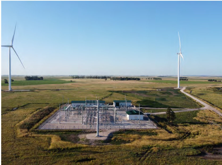
Image 02 – Typical Substation (Source: EMM)
