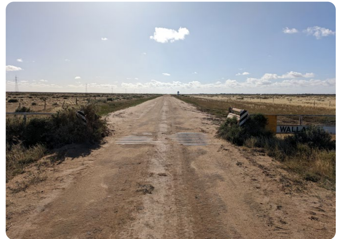
Above: West Burrabogie Rd, showing current condition of road surface, cattle grid and general site terrain characteristics.
