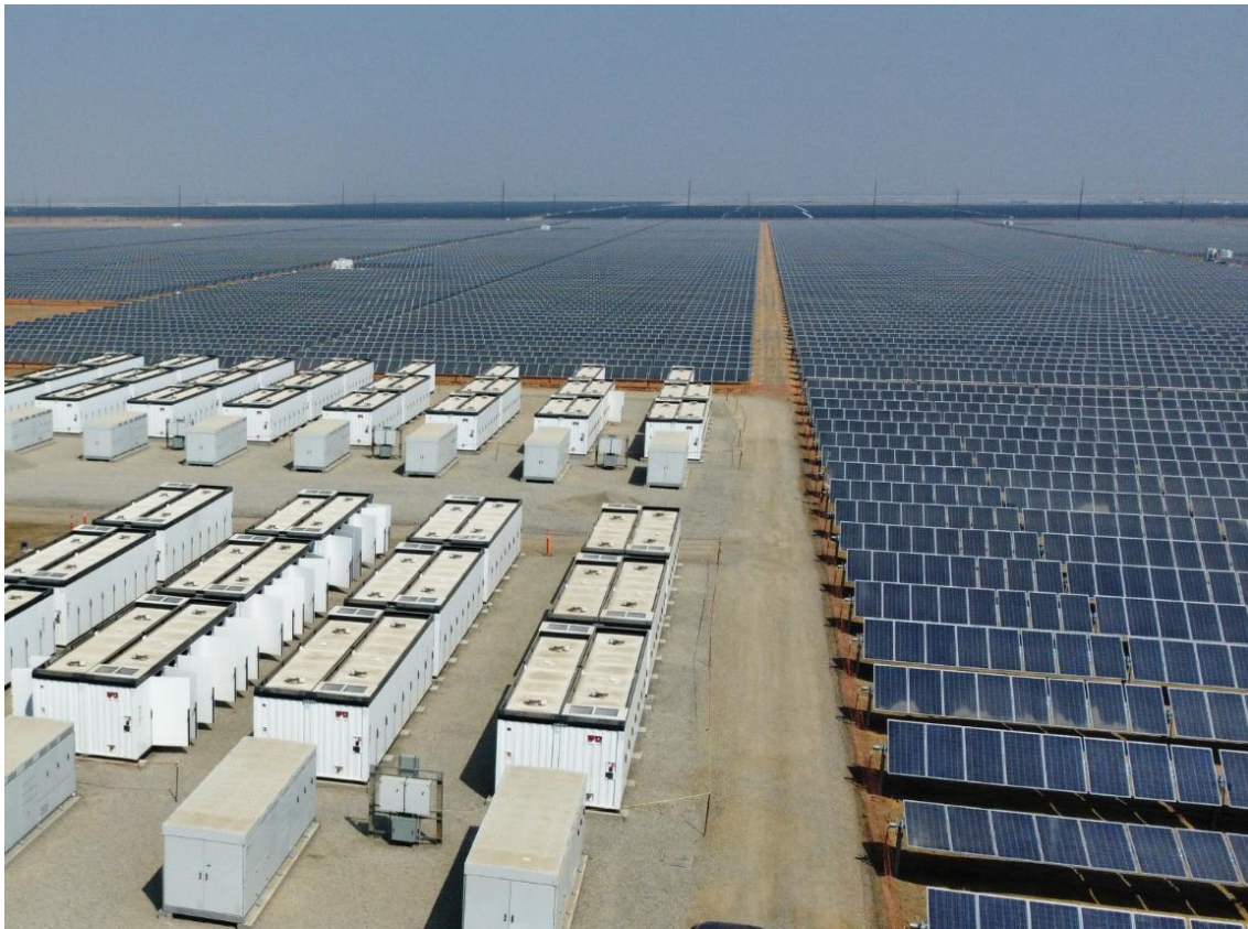
Figure 18 Example CSI SolBank Installations
