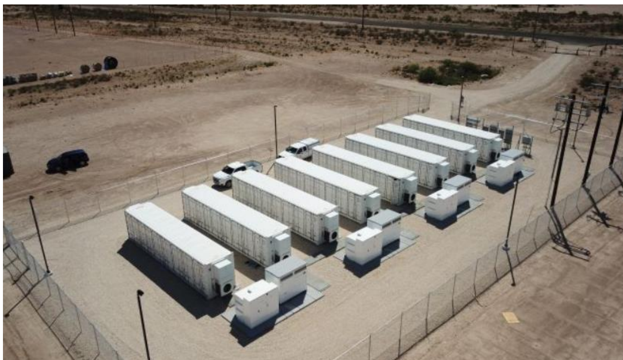
Figure 3-3: Typical Powin BESS Arrangement
