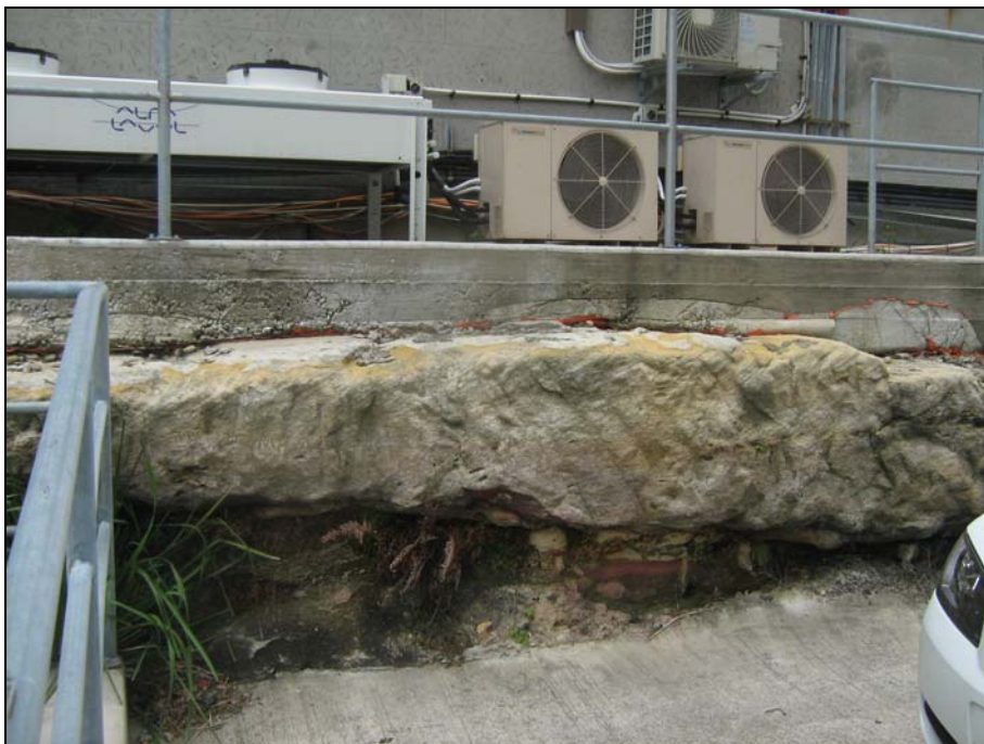
Figure 6. Sandstone exposed by excavation at the base and rear of building adjacent to and at same level as the Blackett building.
