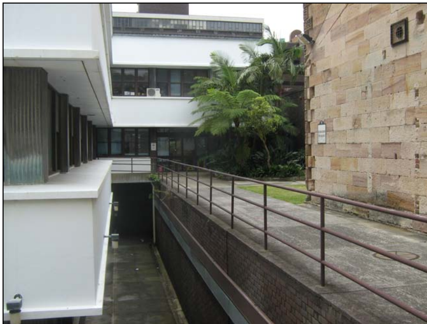
Figure 8. Cutting before the Oncology Building and Blackett Building showing deep excavation below Blackett level and into sandstone bedrock.
