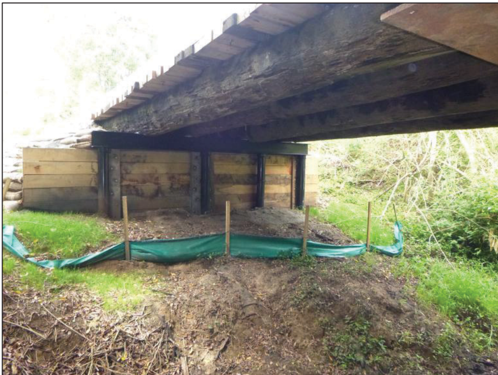
Plate 19: Planking, sandbagging, and a silt fence have been instated to combat erosion at this end of the bridge. Further steel supports can be seen and this type of support exists at the other end of the bridge. Replacement planks are also visible on the underside of the bridge's surface.
