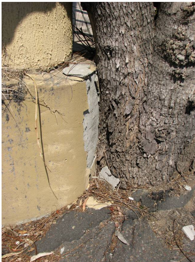
Figure 5: Tree 8 showing how the trunk is compressed against the pier of the existing building.
