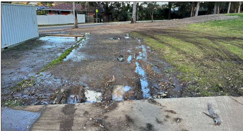
Photograph 5: View of ponded water/rutting to the south of the site looking east
