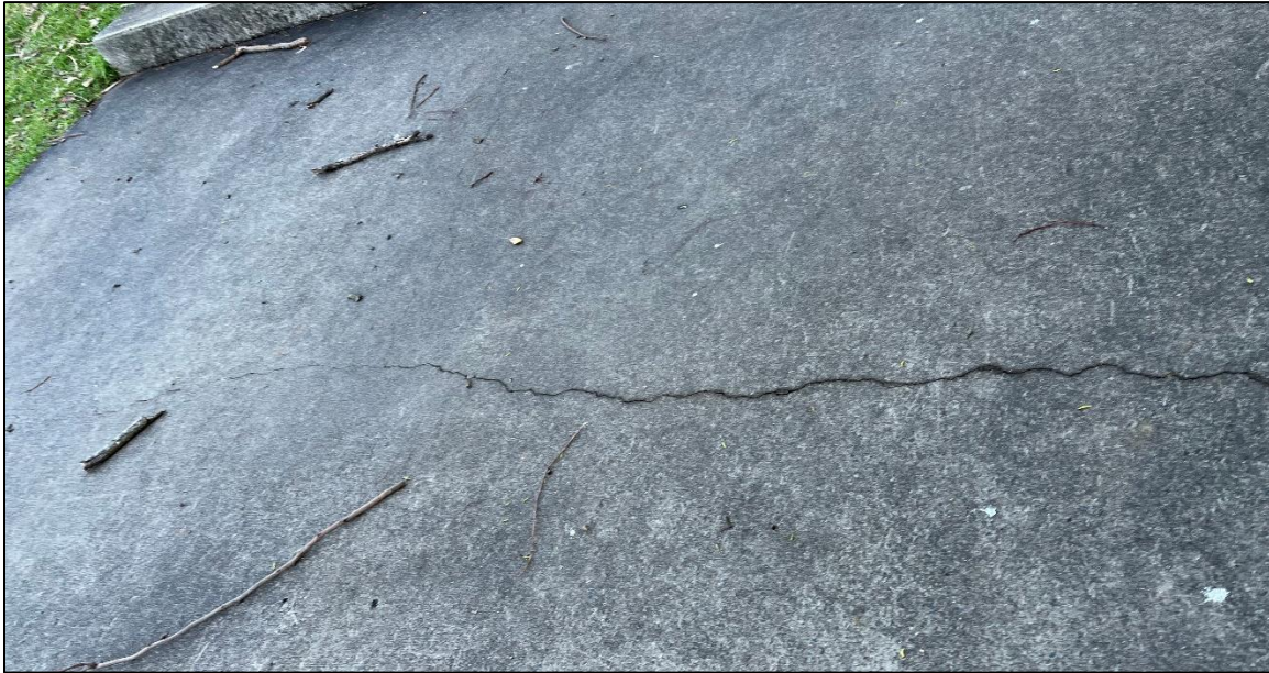
Photograph 4: Views of the cracking in an access ramp to the west of the site
