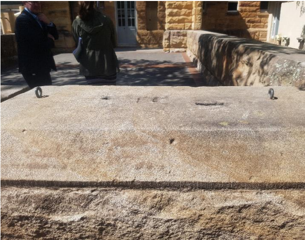
Figure 43 - Rivet impressions within the exposed sandstone blocks hint at the former rough cut sandstone columns of the Fernery which stood in this location
