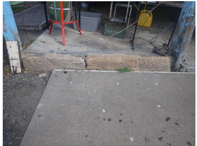
Figure 56 – Sandstone footings identified as having been integrated into a barn associated with the Agricultural Centre.
