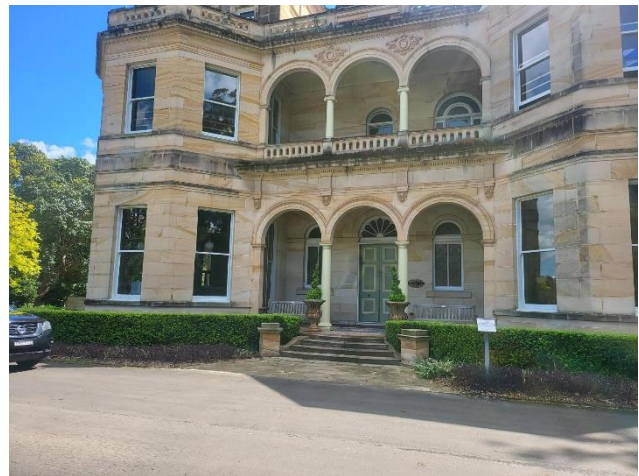
Figure 52 – General view of Gowan Brae, showing the abrupt intrusion of the asphalt onto the sandstone paving at the entryway.
