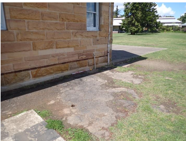
Figure 57 – Potential road surface or flooring identified as exposed to the west of the Stables.
