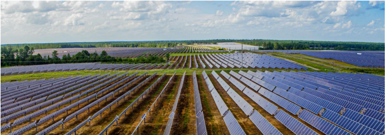
Photo 3.1 Typical solar panel configuration
