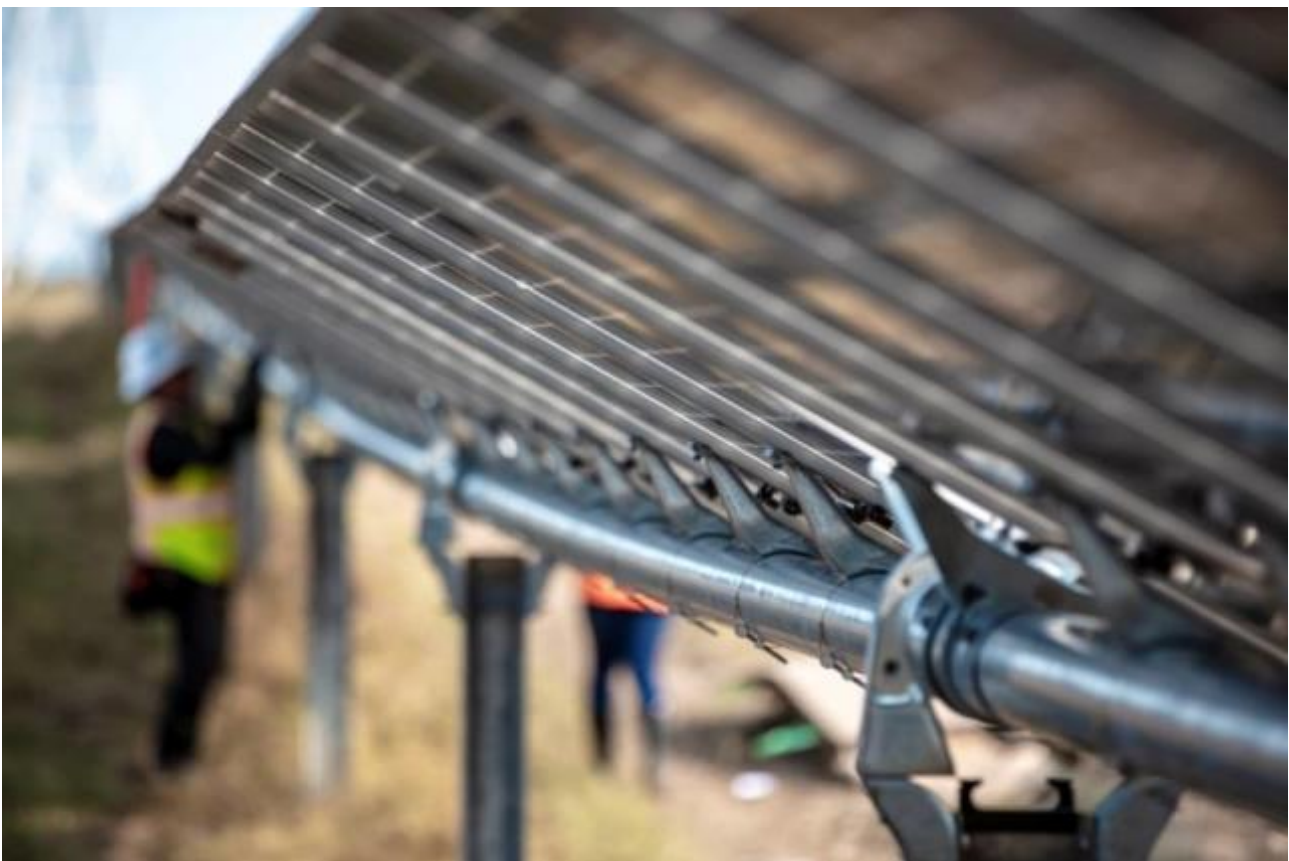
Photo 3.2 Example of Typical Single Axis Tracking System
