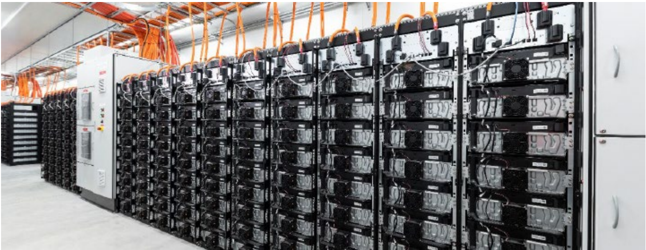
Photograph 3.2 Example of individual battery modules installed in racks and connected via cabling
