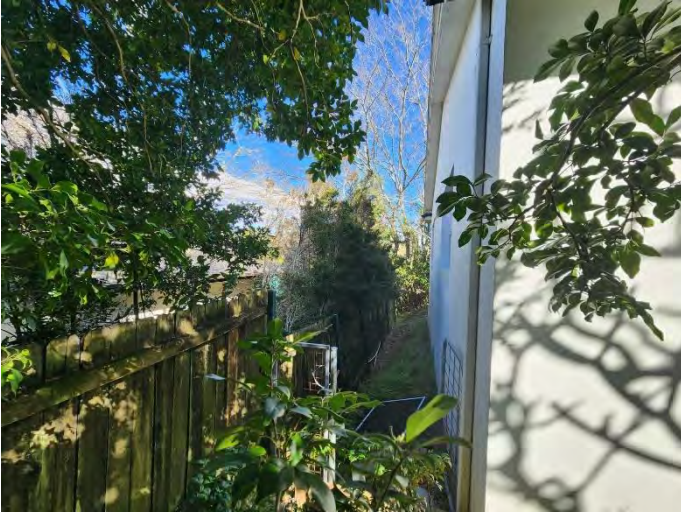
Plate 7 – View along the eastern side of 293 Mona Vale Road. Window frame was found on the ground during the time of site inspection.
