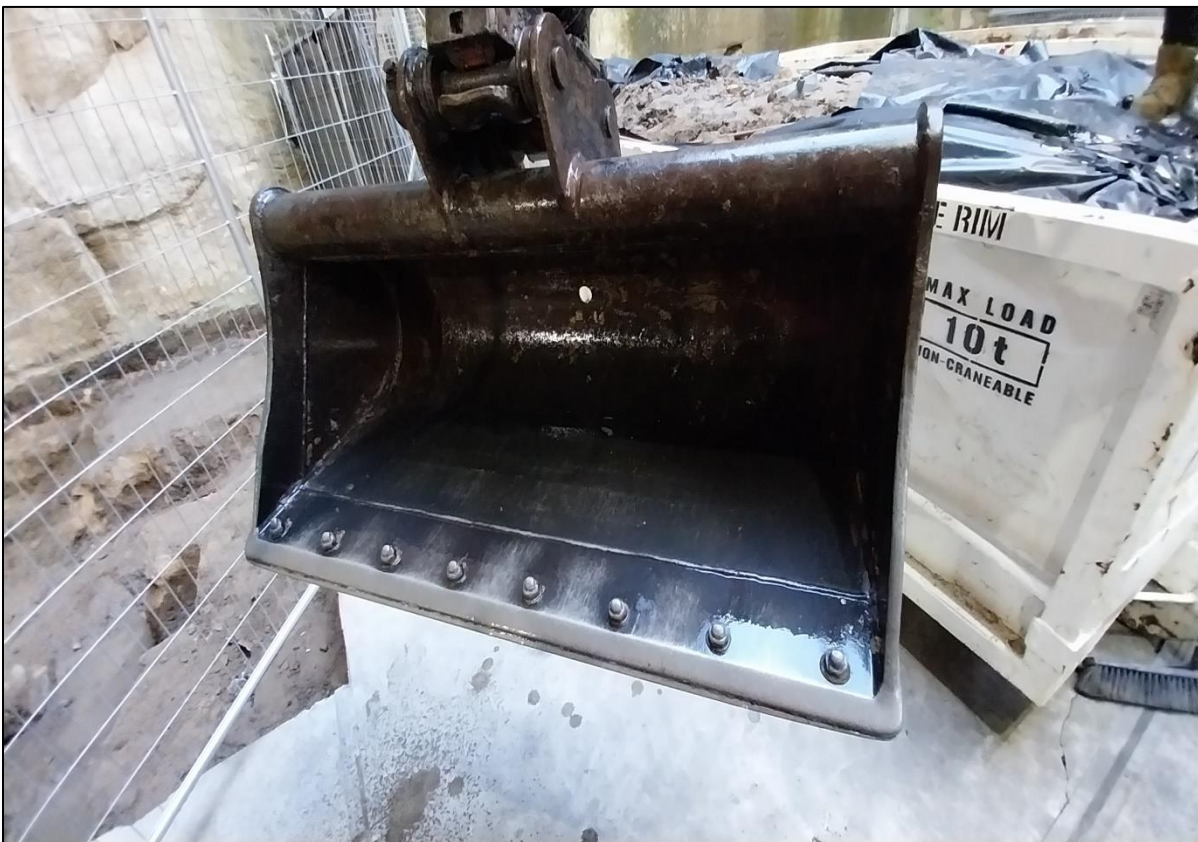
Photograph 4. Subject area 2) - Site interior, northern extent, adjacent rock wall, excavator Kubota U35-4, top of bucket to former asbestos containing soil.
