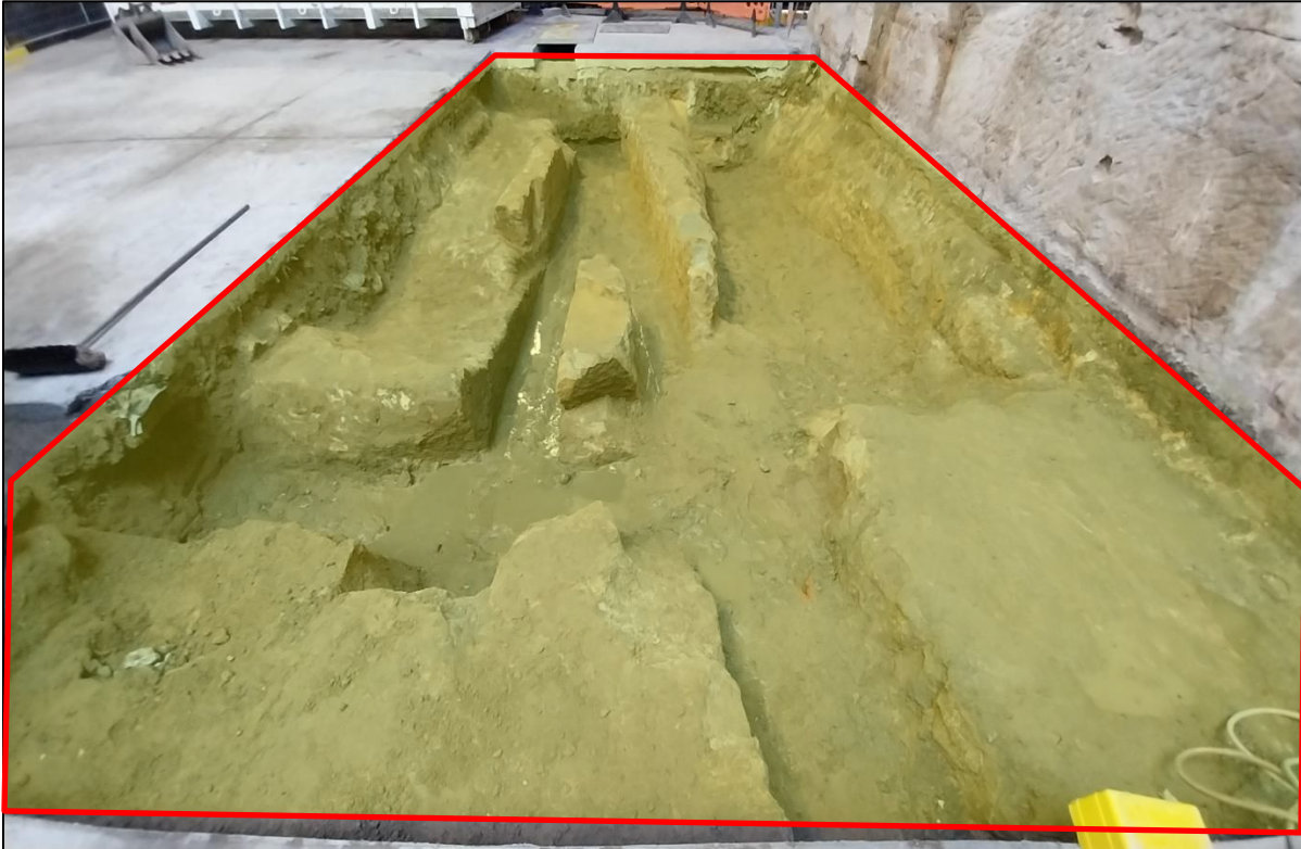
Photograph 3. Subject area 1) - Site interior, northern extent, adjacent rock wall, excavated section of concrete, top of surfaces only to former asbestos containing soil.
