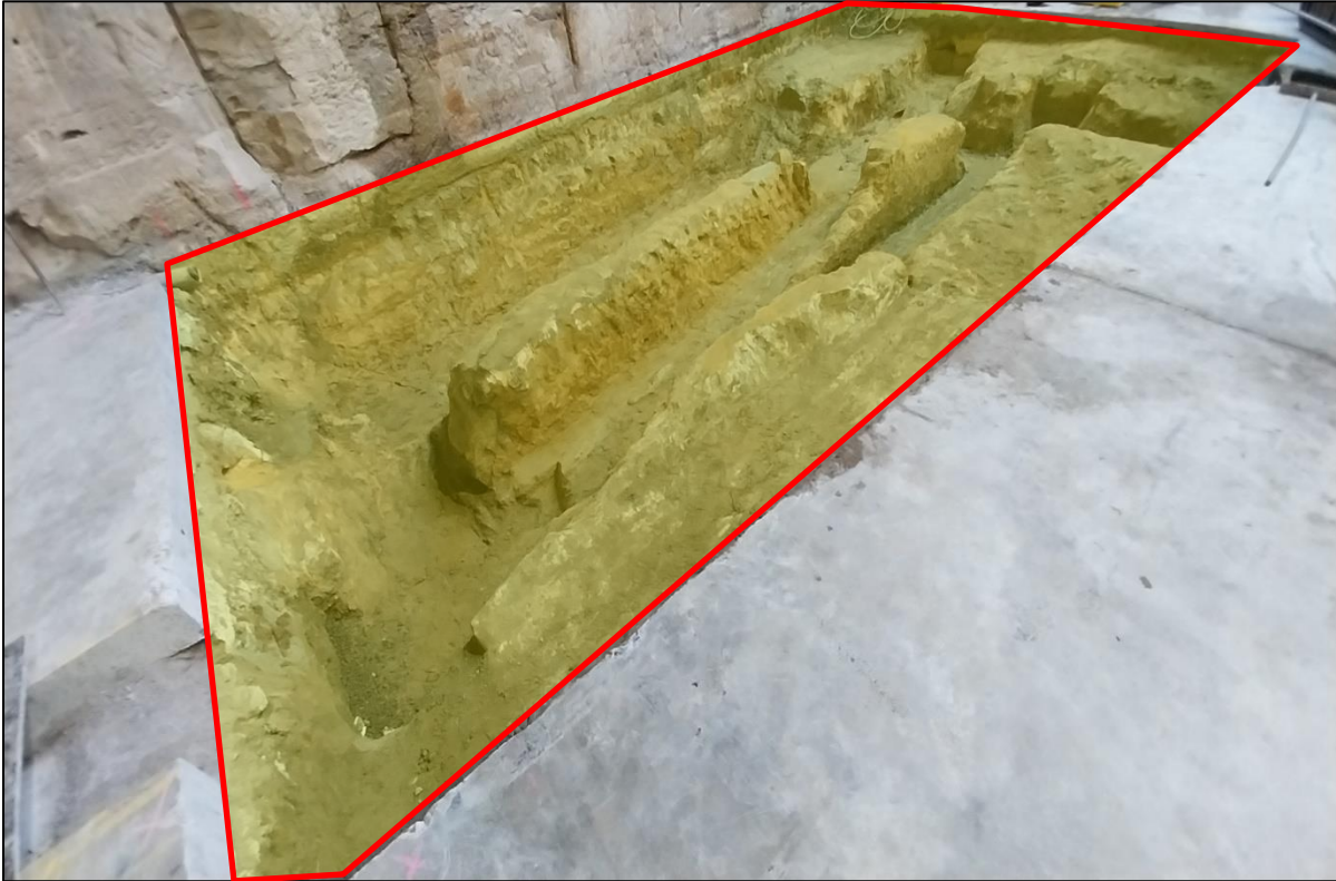
Photograph 1. Subject area 1) - Site interior, northern extent, adjacent rock wall, excavated section of concrete, top of surfaces only to former asbestos containing soil.
