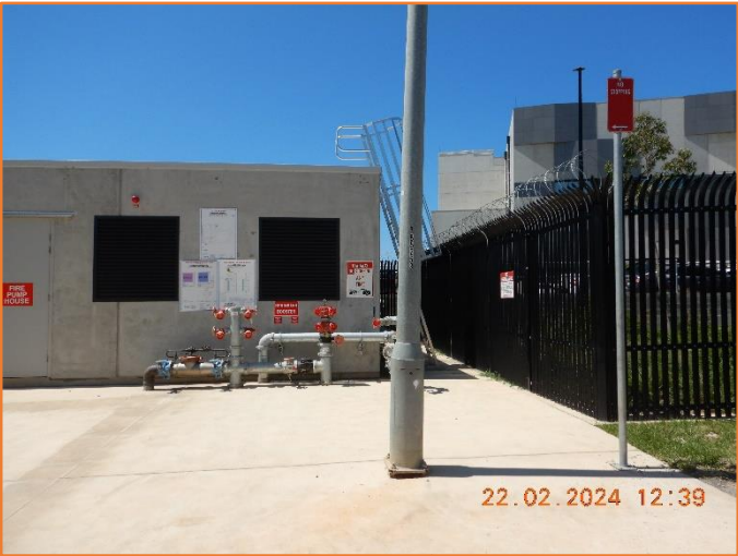
Figure 21: Poor - General condition of monopole assembly. Moderate rotation observed.
