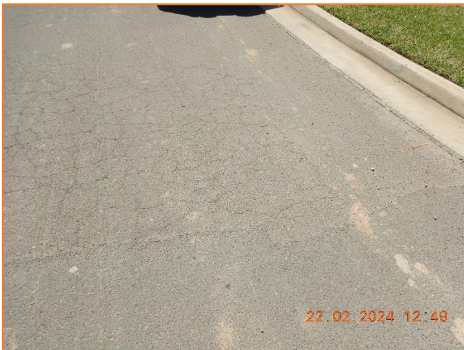
Figure 152: Reasonable - General condition of flexible pavement. Moderate alligator cracking observed.
