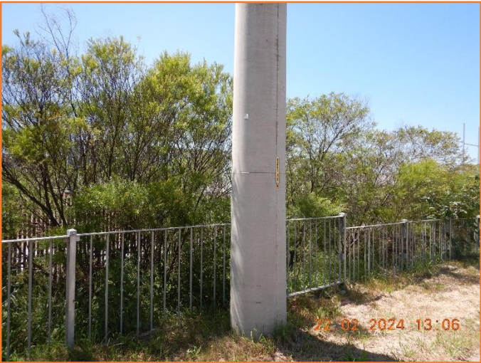
Figure 343: Good - General condition of monopole assembly.
