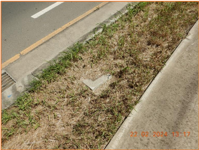
Figure 441: Defective - General condition of service pit.
