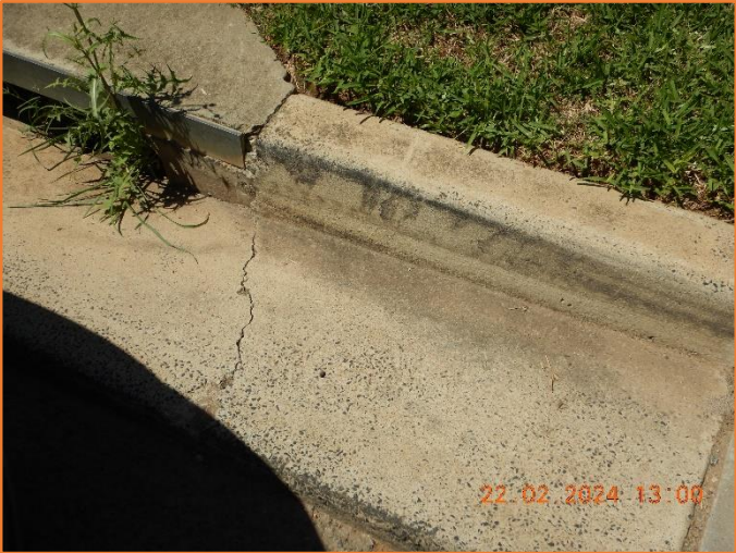
Figure 277: Reasonable - General condition of kerb inlet pit. Moderate cracking observed.
