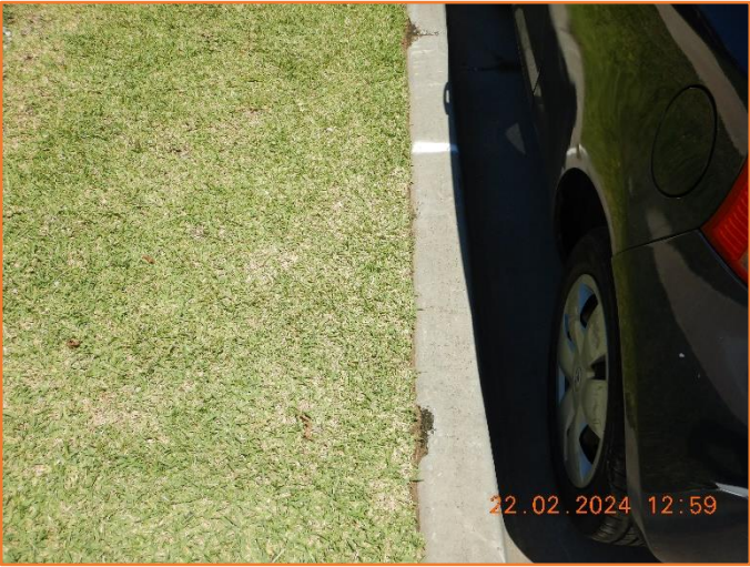
Figure 266: Reasonable - General condition of kerb and gutter. Minor spalling observed.
