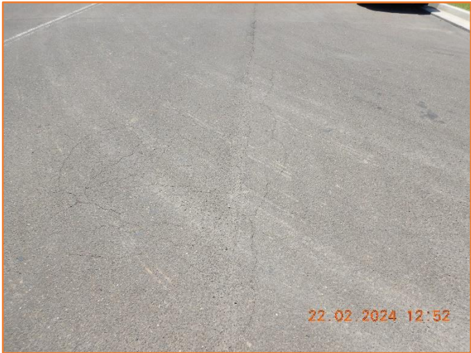
Figure 178: Reasonable - General condition of flexible pavement. Moderate alligator cracking observed.
