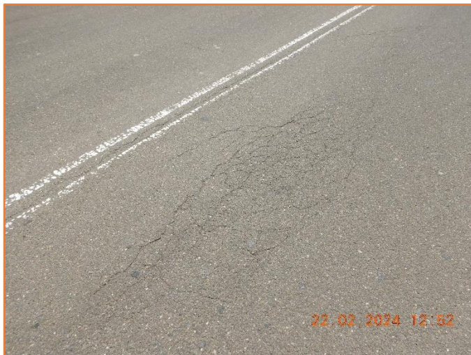
Figure 184: Reasonable - General condition of flexible pavement. Moderate alligator cracking and rutting observed.
