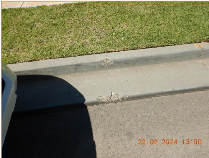
Figure 271: Reasonable - General condition of kerb and gutter. Moderate cracking and spalling observed.
