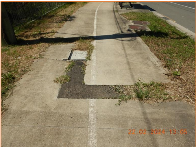
Figure 331: Poor - General condition of footpath. Previous repair works observed.
