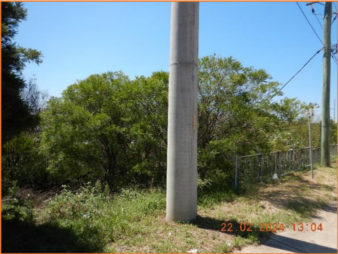
Figure 324: Good - General condition of monopole assembly.
