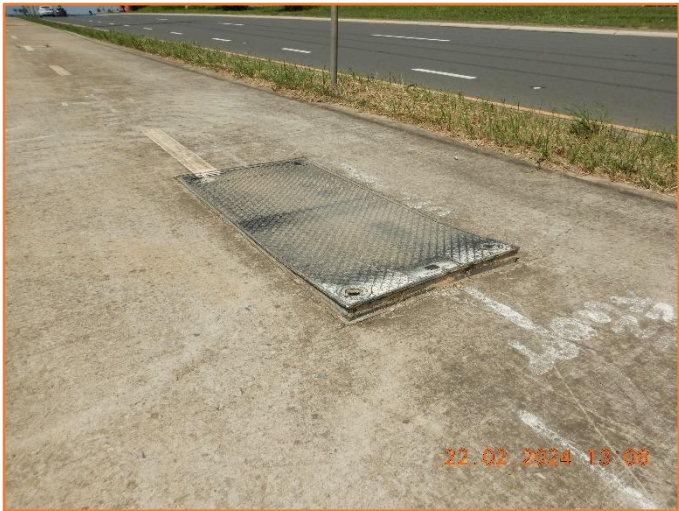
Figure 372: Poor - General condition of service pit. Moderate vertical displacement observed.
