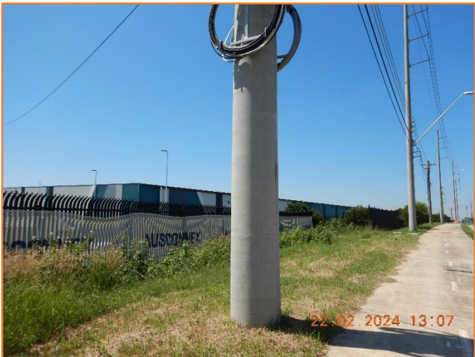
Figure 370: Good - General condition of monopole assembly.
