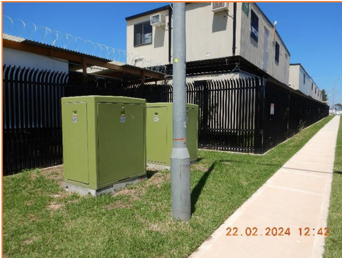
Figure 76: Good - General condition of monopole assembly.
