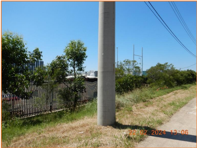
Figure 353: Good - General condition of monopole assembly.
