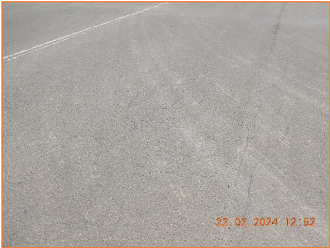
Figure 179: Reasonable - General condition of flexible pavement. Moderate alligator cracking observed.
