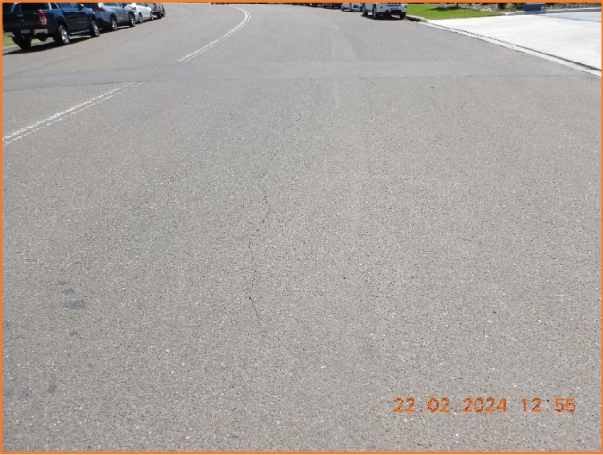
Figure 214: Reasonable - General condition of flexible pavement. Moderate cracking observed.
