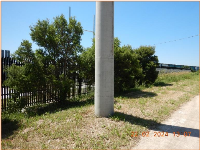
Figure 365: Good - General condition of monopole assembly.
