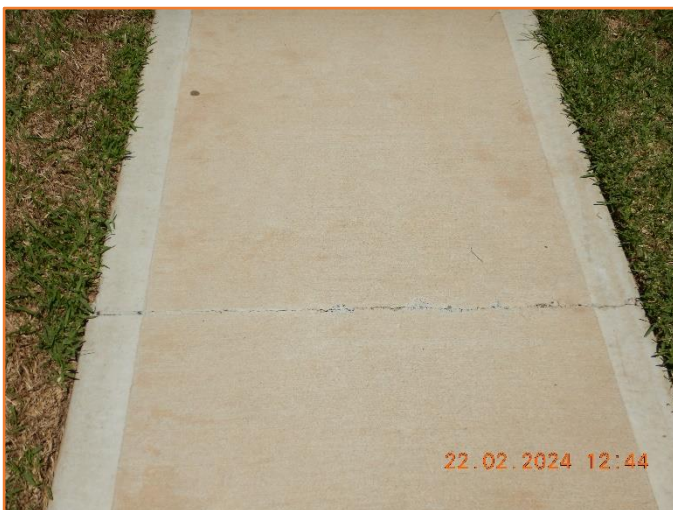
Figure 95: Reasonable - General condition of footpath. Moderate hairline cracking observed.
