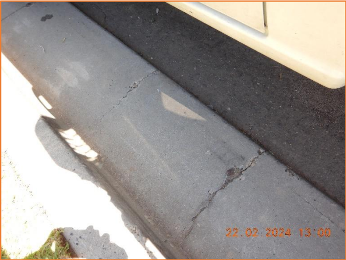
Figure 269: Reasonable - General condition of kerb and gutter. Moderate cracking observed.
