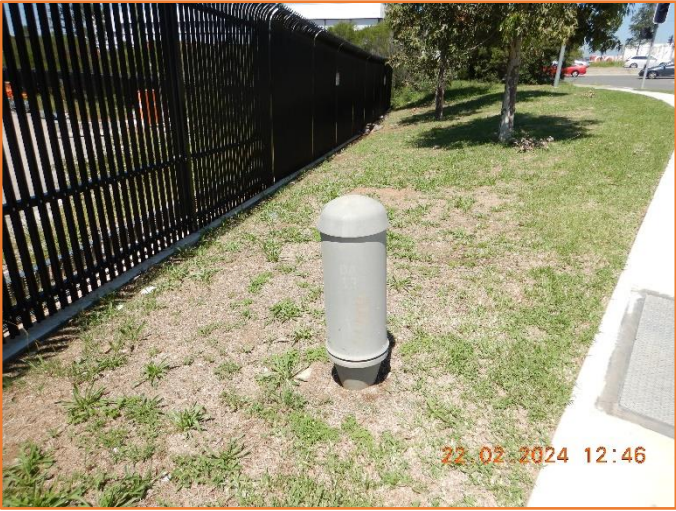
Figure 119: Reasonable - General condition of substation.
