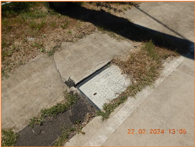
Figure 333: Poor - General condition of footpath and service pit. Moderate cracking observed.
