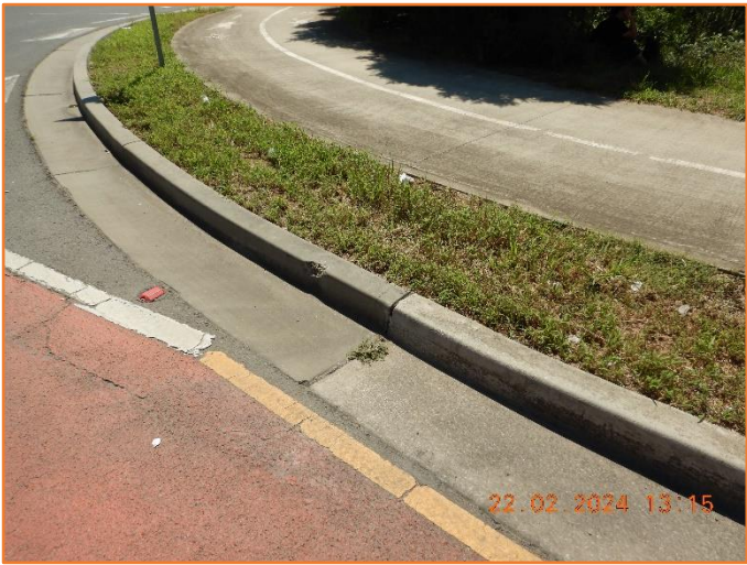
Figure 423: Reasonable - General condition of kerb and gutter. Moderate spalling observed.
