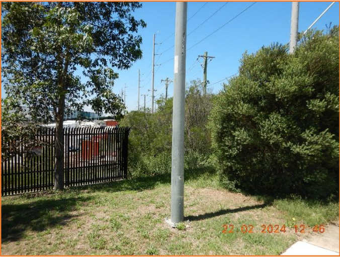
Figure 131: Good - General condition of monopole assembly.
