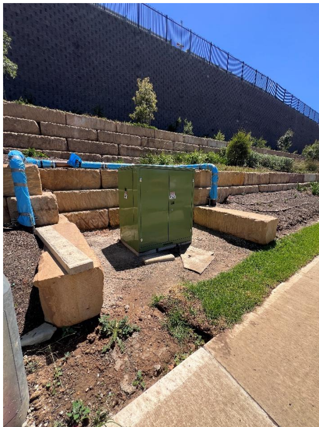
Figure 8 – General condition of the electrical box / junction box.
