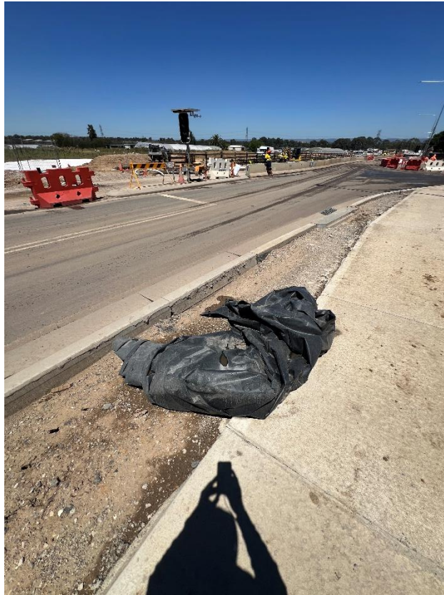
Figure 19 – General condition of the kerb.
