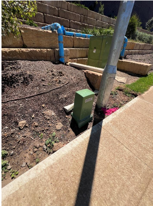
Figure 9 – General condition of the electrical box / junction box.
