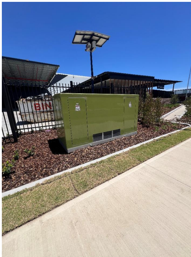
Figure 246 – General condition of the electrical box / junction box.
