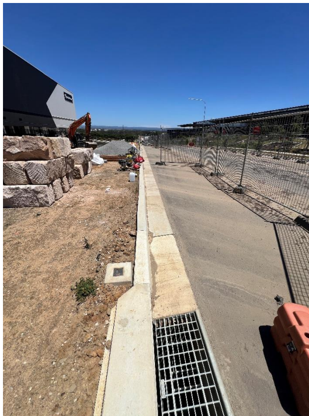
Figure 268 – General condition of the drain.
