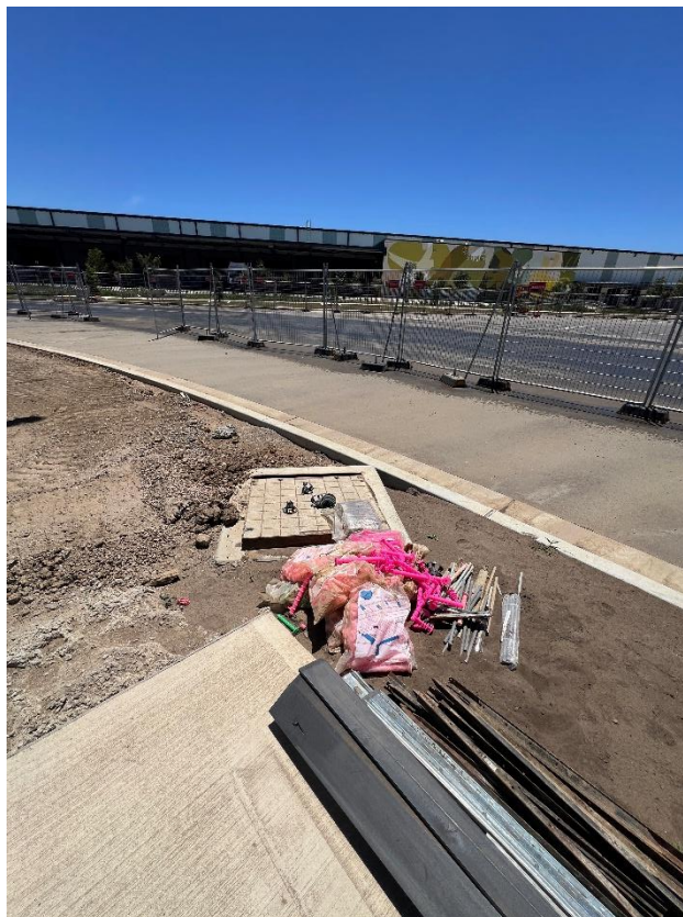
Figure 252 – Some areas were not inspected due to the presence of stored materials.
