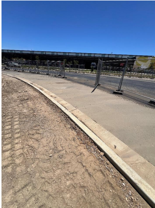
Figure 255 – General condition of the kerb.
