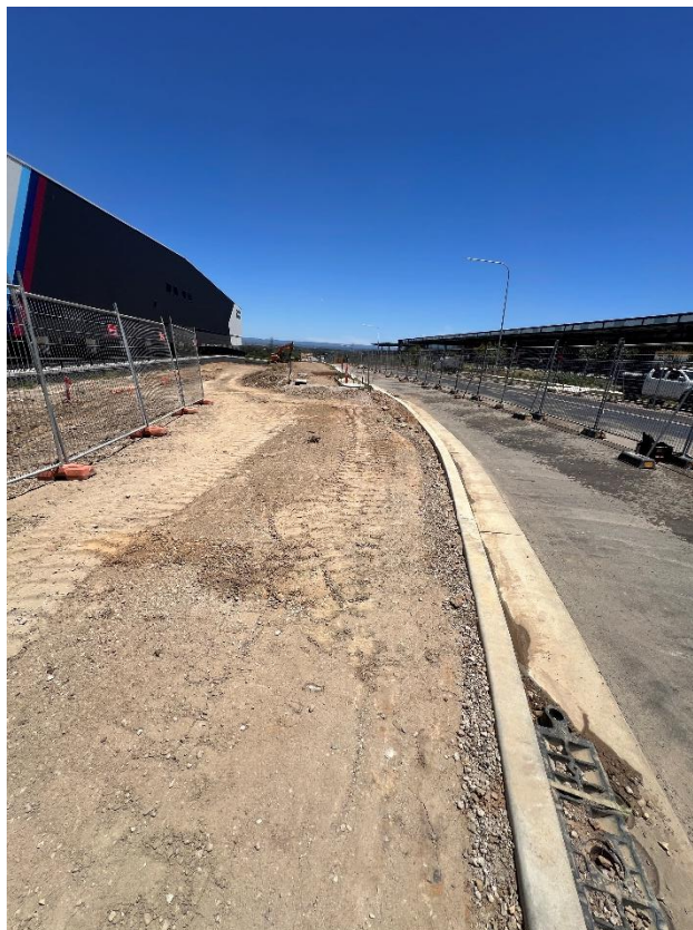
Figure 258 – General condition of the kerb.
