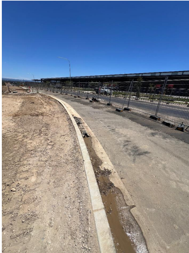
Figure 257 – General condition of the kerb.
