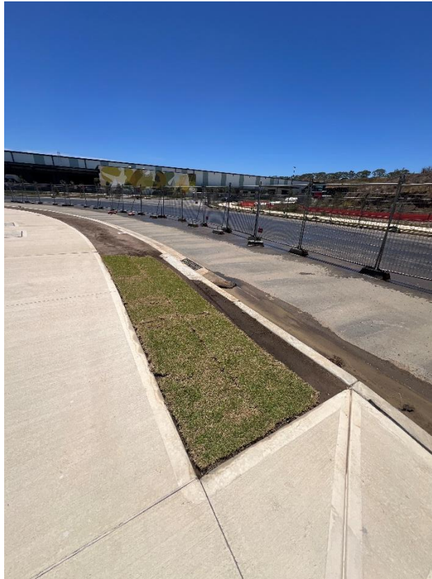
Figure 247 – General condition of the kerb.
