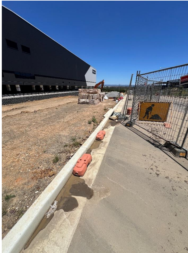
Figure 267 – General condition of the kerb.
