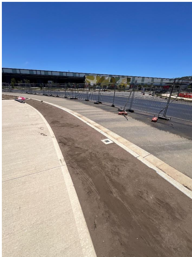
Figure 250 – General condition of the kerb.
