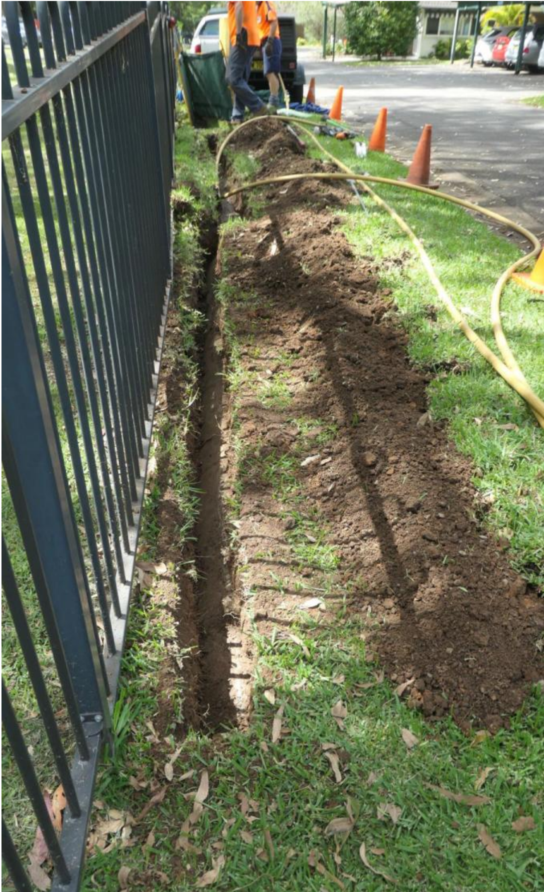
Figure 6 – Photo of the area where root investigations were carried out. Trench depth and depth of investigation was dictated by presence of large concrete stormwater pipe. The northern side of pipe was exposed and investigated where possible to check for any roots tracking along the pipe run. None were observed. (Photo: Arterra 16/2/22)
