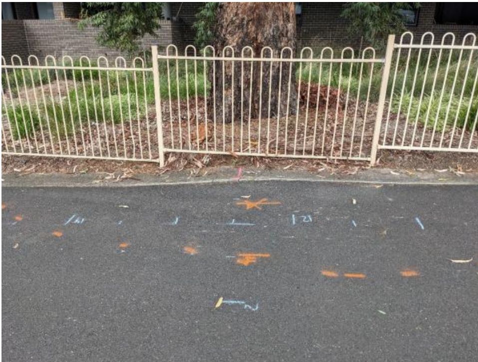
Figure 3. Site image looking towards tree T76 and the area of ground deformation. The dashed orange lines outline the extent of the deformation.
