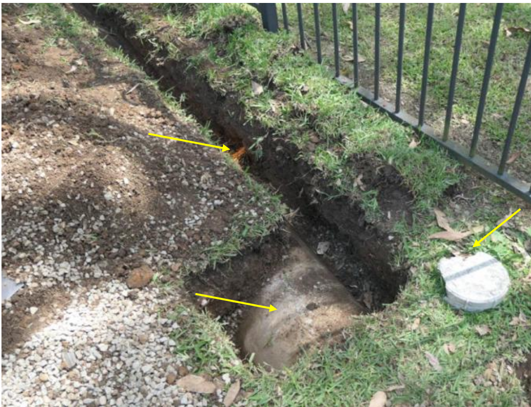
Figure 5 – Photo of the area where root investigations were carried out. Line of trench and depth in some areas of the investigation were dictated by the presence of a large concrete stormwater pipe. The northern side of pipe was exposed where possible to check for any roots tracking along pipe run. Only one very small root was observed in any of the trenching. Note the riser cap from the lower sewer line which was running alongside and lower than the stormwater line. The small root, stormwater pipe and sewer shown arrowed. (Photo: Arterra 16/2/22)
