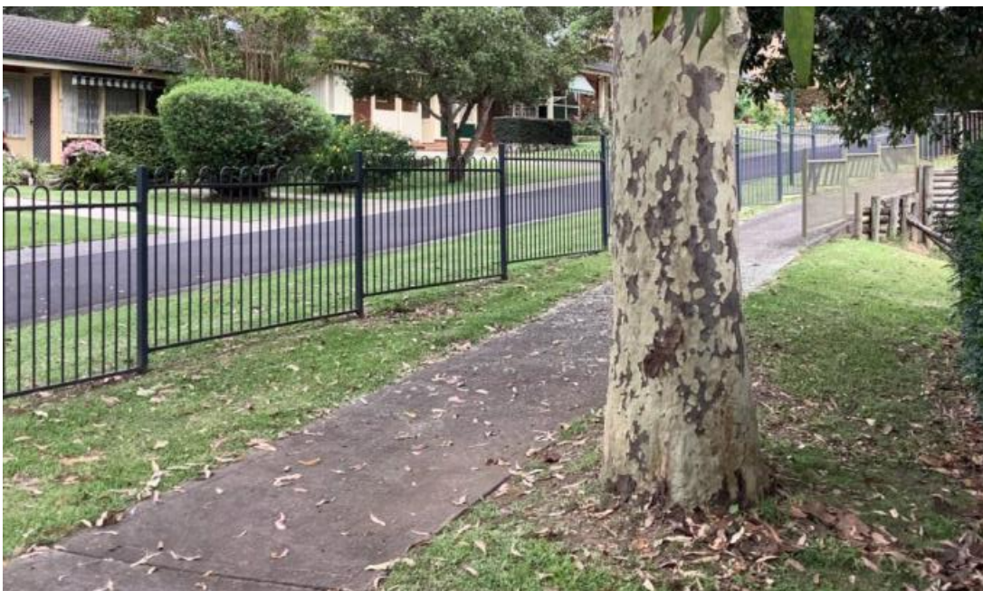
Figure 1 – Photo of the base of Tree T05 Corymbia maculata with existing concrete footpath shown close to the base of the tree. (Photo: Arterra 11/12/21)
