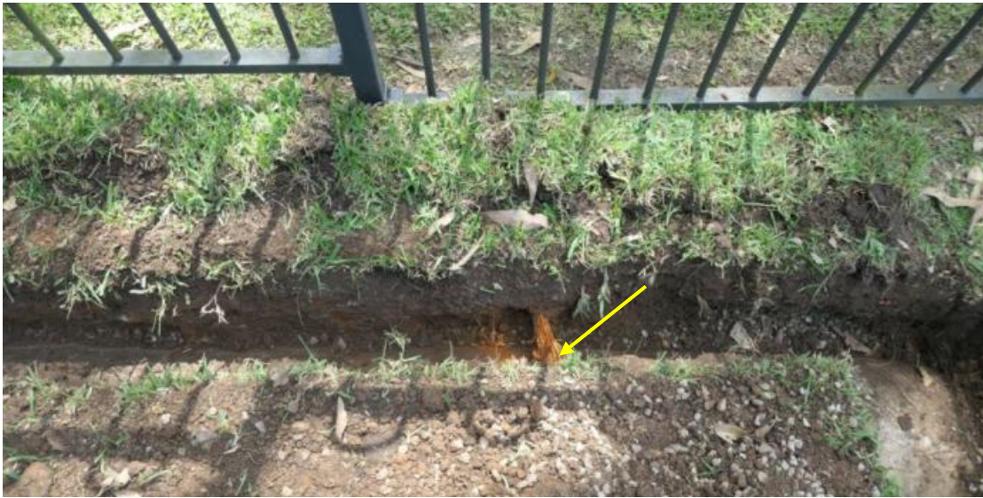
Figure 7 – Only one very small root (20mm \phi ) was discovered along the entire length of the trench. The root was spray painted orange for visibility and shown arrowed. (Photo: Arterra 16/2/22)
