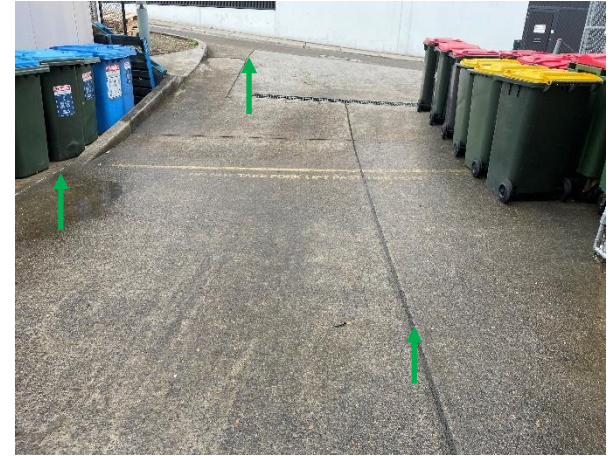
Photo 3: External – Non-asbestos containing bituminous mastic and grey mastic to loading dock and footpath expansion joint.
