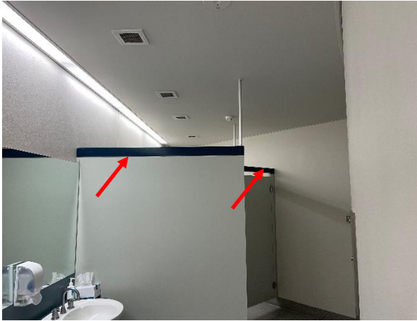
Photo 13: Ground – Lead based blue paint to metal rail over toilet cubical within the male bathroom
