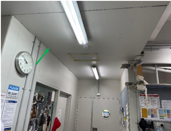
Photo 10: Ground – Non-asbestos containing fibre cement sheeting to ceiling cable runner within the loading dock
