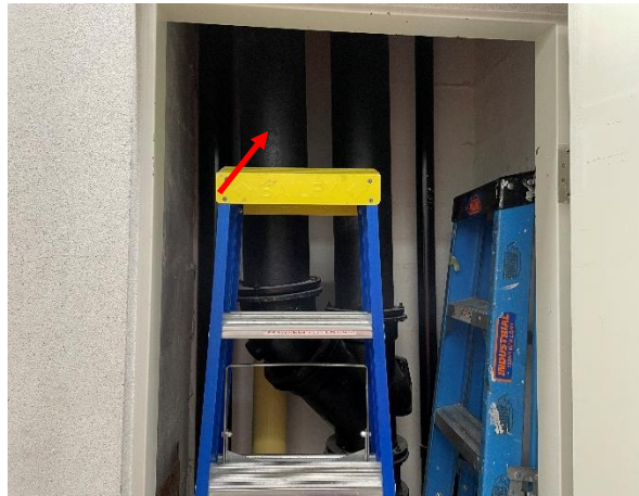
Photo 17: Level 1 – Lead based black paint to metal sewer pipework
