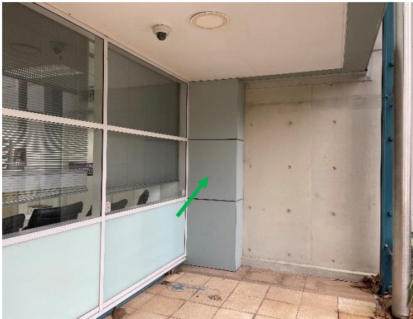
Photo 4: External – Non-asbestos containing fibre cement grey sheet cladding panel to the southeast interface of Research building and Ainsworth building
