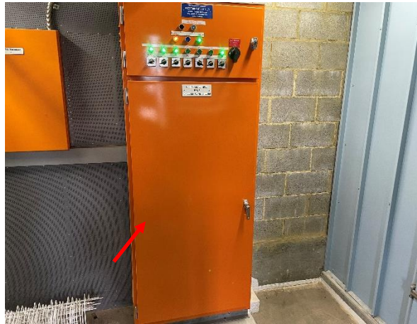
Photo 23: Roof – Assumed lead based orange paint to electrical distribution box
