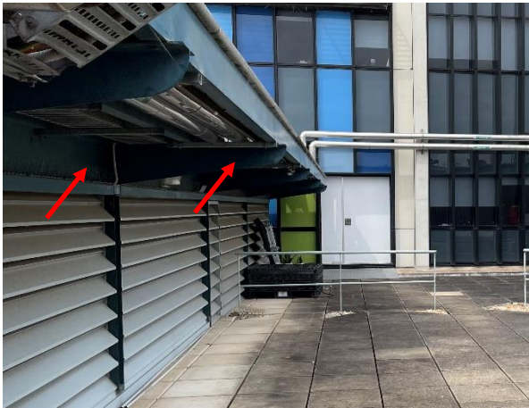
Photo 22: Roof – Lead based blue paint to metal framework of building
