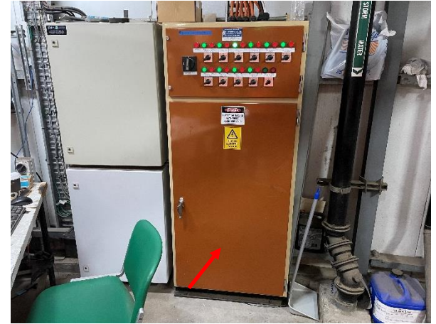
Photo 21: Roof – Lead based brown paint to electrical distribution box within the central plant room
