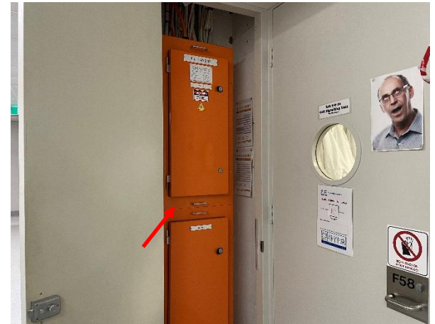
Photo 18: Level 1 – Assumed lead based orange paint to electrical distribution box
