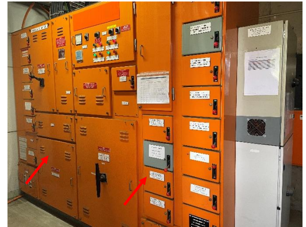
Photo 12: Ground – Assumed lead based orange paint to electrical distribution box
