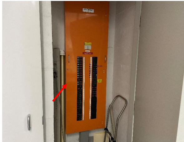
Photo 11: Ground – Lead based orange paint to electrical distribution box
