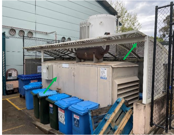
Photo 2: External – Non-asbestos containing grey mastic seals to generator and non-lead based cream paint to generator shed.
