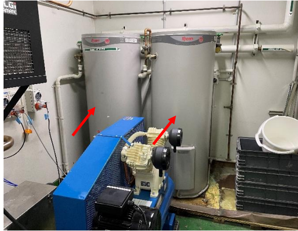
Photo 14: Ground – Assumed SMF internal insulation to hot water units within room G53
