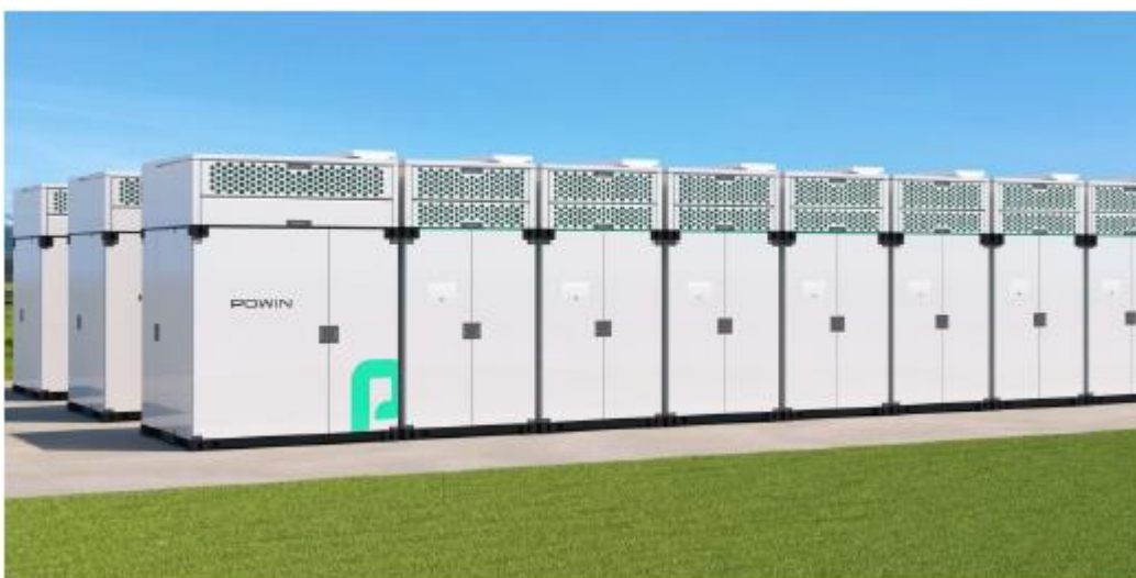
Figure 3-4 Example of a typical battery unit (Powin Centipede Platform with Stack750E)
