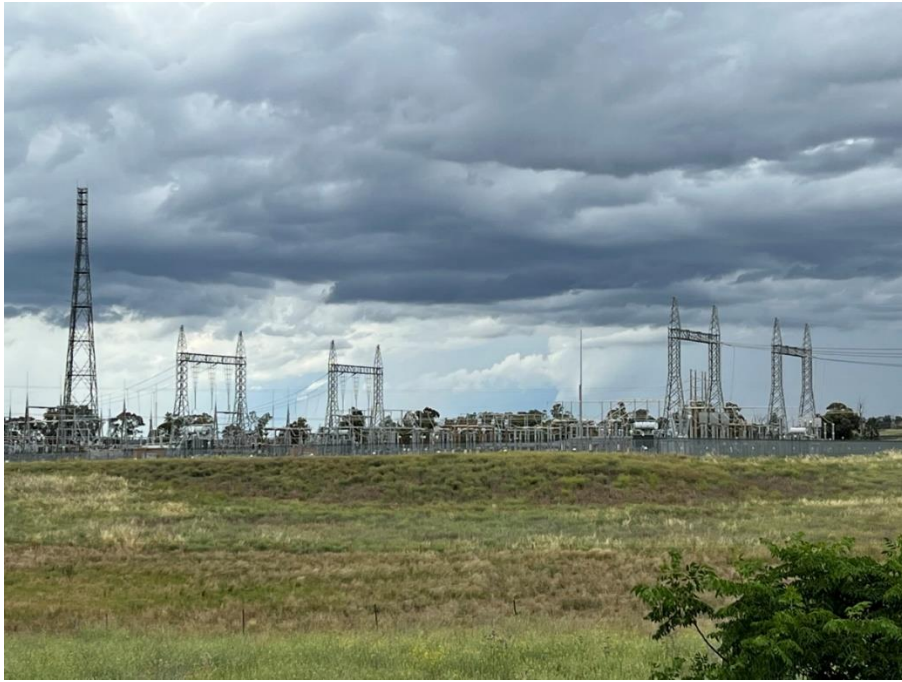
E3 Existing 330kV substation (Wellington Substation) (looking to the north at the southern boundary of the substation from the Development footprint)
