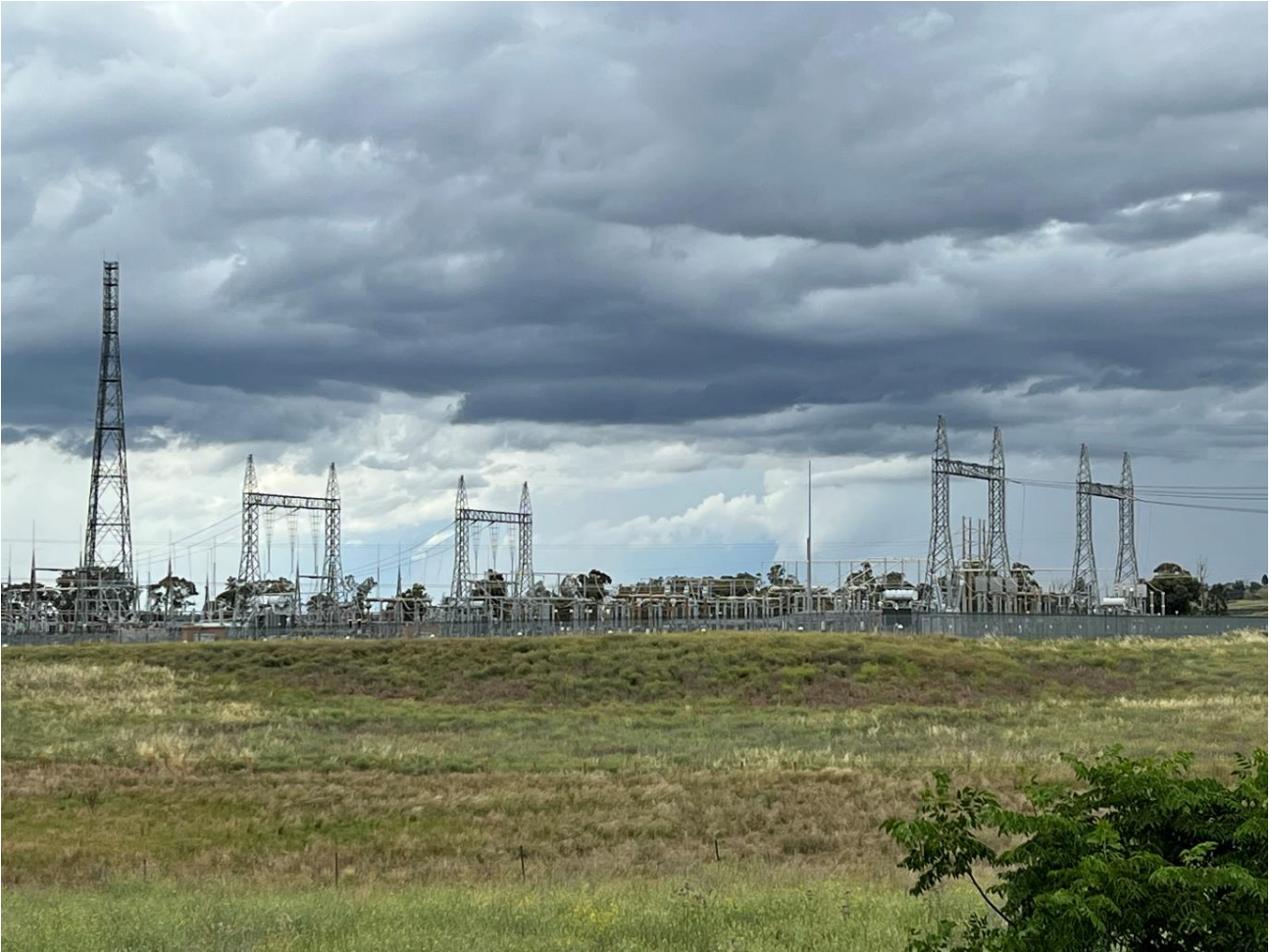
Figure 3-6 Existing 330kV substation (Wellington Substation) (looking to the north at the southern boundary of the substation from the Development Footprint)
