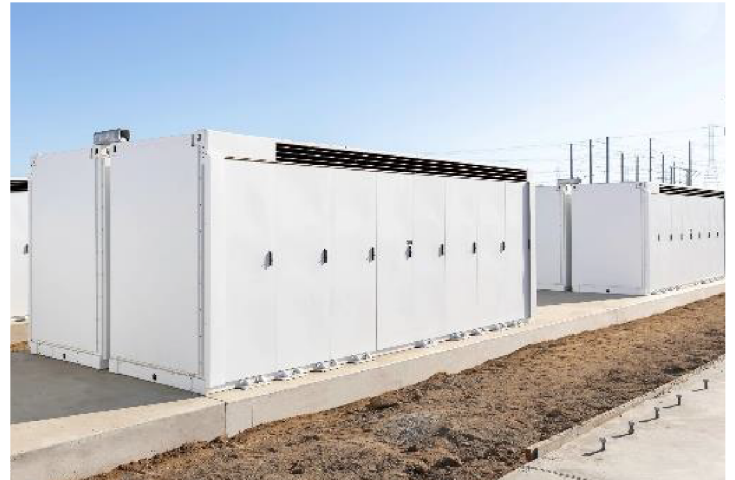
Example of a typical BESS
