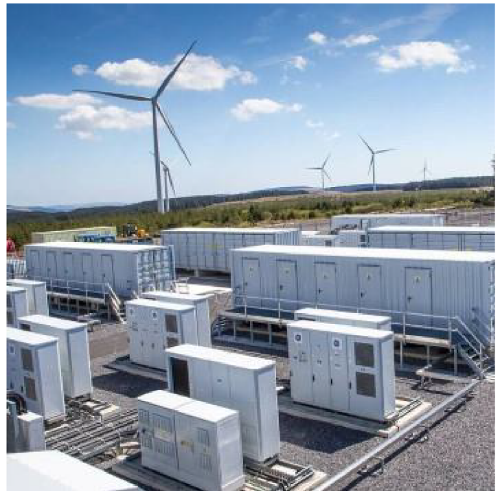
Example of a typical BESS
