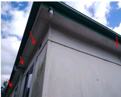
Photo No: 221107-100836 Result: Asbestos - Presumed Positive Location-Level: Exterior - Ground Floor Room-Location: All elevation of the building - eaves Feature-Material: FC sheeting Item No - Risk Rating: 19 - Low
