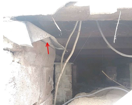
Photo No: 221107-100951 Result: Asbestos - Positive Location-Level: Interior - Ground Floor Room-Location: All elevation of the building - packer Feature-Material: FC sheeting Item No - Risk Rating: 20 - Low
