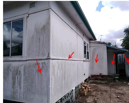
Photo No: 221107-100910 Result: Asbestos - Positive Location-Level: Exterior - Ground Floor Room-Location: All elevation of the building - walls Feature-Material: FC sheeting Item No - Risk Rating: 18 - Medium
