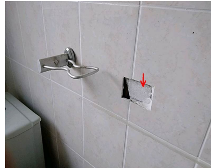
Photo No: 221107-094420 Result: Asbestos - Positive Location-Level: Interior - Ground Floor Room-Location: Bathroom - walls (behind tiles) Feature-Material: FC sheeting Item No - Risk Rating: 5 - Medium
