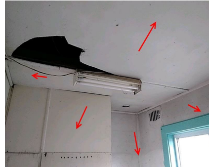
Photo No: 221107-100520 Result: Asbestos - Presumed Positive Location-Level: Exterior - Ground Floor Room-Location: Laundry - internal walls and ceiling Feature-Material: FC sheeting Item No - Risk Rating: 16 - Medium
