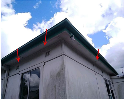
Photo No: 221107-101245 Result: Asbestos - Presumed Positive Location-Level: Exterior - Ground Floor Room-Location: All elevation of the building - eaves Feature-Material: FC sheeting Item No - Risk Rating: 21 - Low
