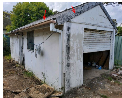
Photo No: 221107-120202 Result: Asbestos - Presumed Positive Location-Level: Exterior - Ground Floor Room-Location: All elevation of garage - roof and verge Feature-Material: FC sheeting Item No - Risk Rating: 3 - Low
