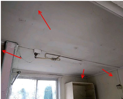
Photo No: 221107-100527 Result: Asbestos - Presumed Positive Location-Level: Exterior - Ground Floor Room-Location: Toilet - internal walls and ceiling Feature-Material: FC sheeting Item No - Risk Rating: 17 - Medium
