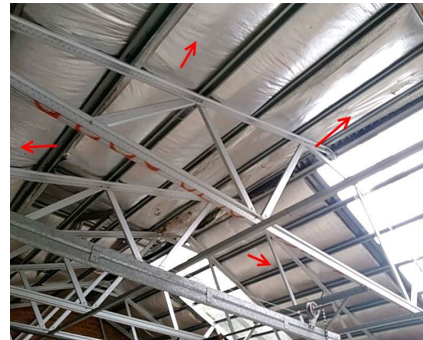
Photo No: 221107-140243 Result: SMF - Positive Location-Level: Interior - Ground Floor Room-Location: All elevation of the roof - sarking Feature-Material: sarking Item No - Risk Rating: 1 -
