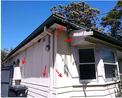
Photo No: 221107-140141 Result: Asbestos - Positive Location-Level: Exterior - Ground Floor Room-Location: All elevation of the building - walls and eaves Feature-Material: FC sheeting Item No - Risk Rating: 8 - Low
