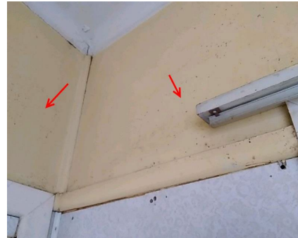
Photo No: 221107-095147 Result: Asbestos - Presumed Positive Location-Level: Interior - Ground Floor Room-Location: Kitchen - walls (behind splashback) Feature-Material: FC sheeting Item No - Risk Rating: 9 - Low
