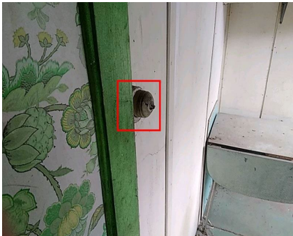
Photo No: 221107-102641 Result: Asbestos - Presumed Positive Location-Level: Interior - Ground Floor Room-Location: Laundry - electrical power switch Feature-Material: Internal insulation Item No - Risk Rating: 26 - Low
