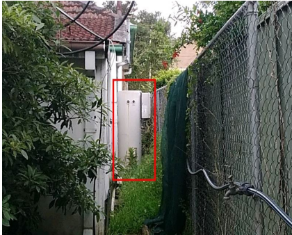
Photo No: 221107-100413 Result: Asbestos - Presumed Positive Location-Level: Exterior - Ground Floor Room-Location: Northern elevation of building - hot water system Feature-Material: Internal insulation Item No - Risk Rating: 15 - Low
