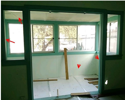
Photo No: 221107-093754 Result: Asbestos - Positive Location-Level: Interior - Ground Floor Room-Location: Living area - sun room Feature-Material: FC sheeting Item No - Risk Rating: 3 - Low
