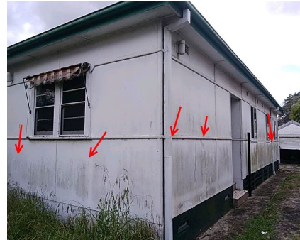
Photo No: 221107-101426 Result: Lead in Paint - Positive Location-Level: Exterior - Ground Floor Room-Location: All elevation of the building - walls and downpipes Feature-Material: Lower colour paint system Item No - Risk Rating: 22 -
