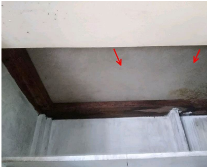
Photo No: 221107-095042 Result: Asbestos - Presumed Positive Location-Level: Interior - Ground Floor Room-Location: Kitchen - cupboard ceiling Feature-Material: FC sheeting Item No - Risk Rating: 8 - Low
