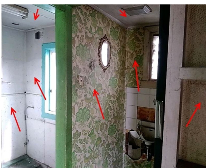
Photo No: 221107-095647 Result: Asbestos - Presumed Positive Location-Level: Exterior - Ground Floor Room-Location: Laundry and toilet - internal walls and ceilings Feature-Material: FC sheeting Item No - Risk Rating: 13 - Low
