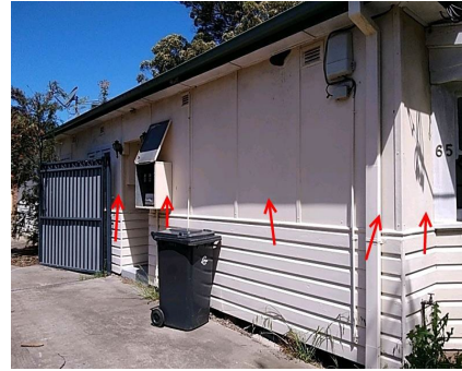
Photo No: 221107-140655 Result: Lead in Paint - Positive Location-Level: Exterior - Ground Floor Room-Location: All elevation of the building - walls Feature-Material: Lower colour paint system Item No - Risk Rating: 10 - Low
