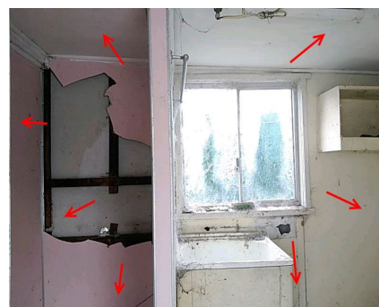
Photo No: 221107-095828 Result: Asbestos - Positive Location-Level: Interior and Exterior - Ground Floor Room-Location: Bathroom - internal walls and ceilings Feature-Material: FC sheeting Item No - Risk Rating: 14 - Medium
