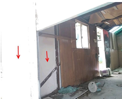
Photo No: 221107-103808 Result: Asbestos - Presumed Positive Location-Level: Interior and Exterior - Ground Floor Room-Location: All elevation of the garage - walls Feature-Material: FC sheeting Item No - Risk Rating: 2 - Low
