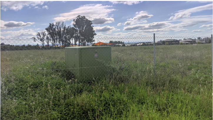
Existing electrical sub station (South east of site) Existing electrical sub station located within the site boundary to be retained and protected in accordance with electrical engineering advice.
