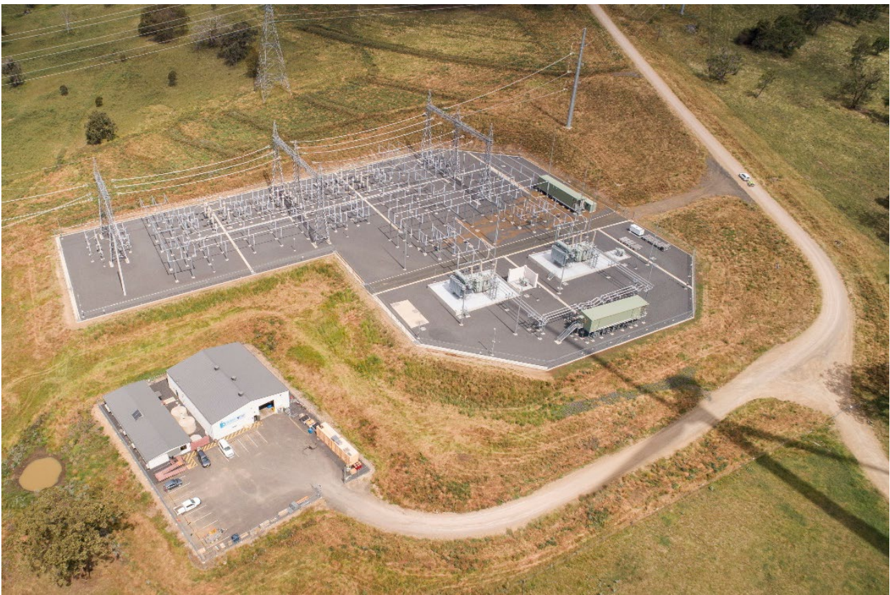
Figure 3.3 Example of an O&M compound and 330 kV/33 kV substation (Sapphire Wind Farm)
