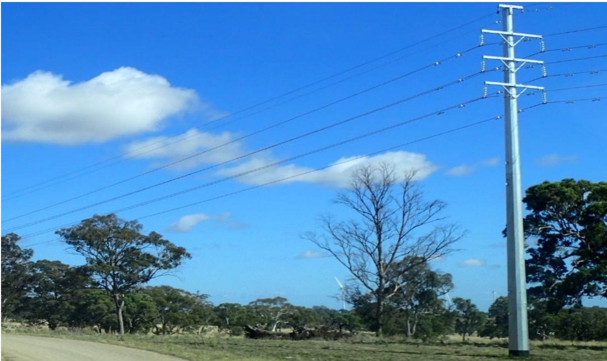
Figure 3.5 Example of a Double-circuit overhead 33 kV transmission line
