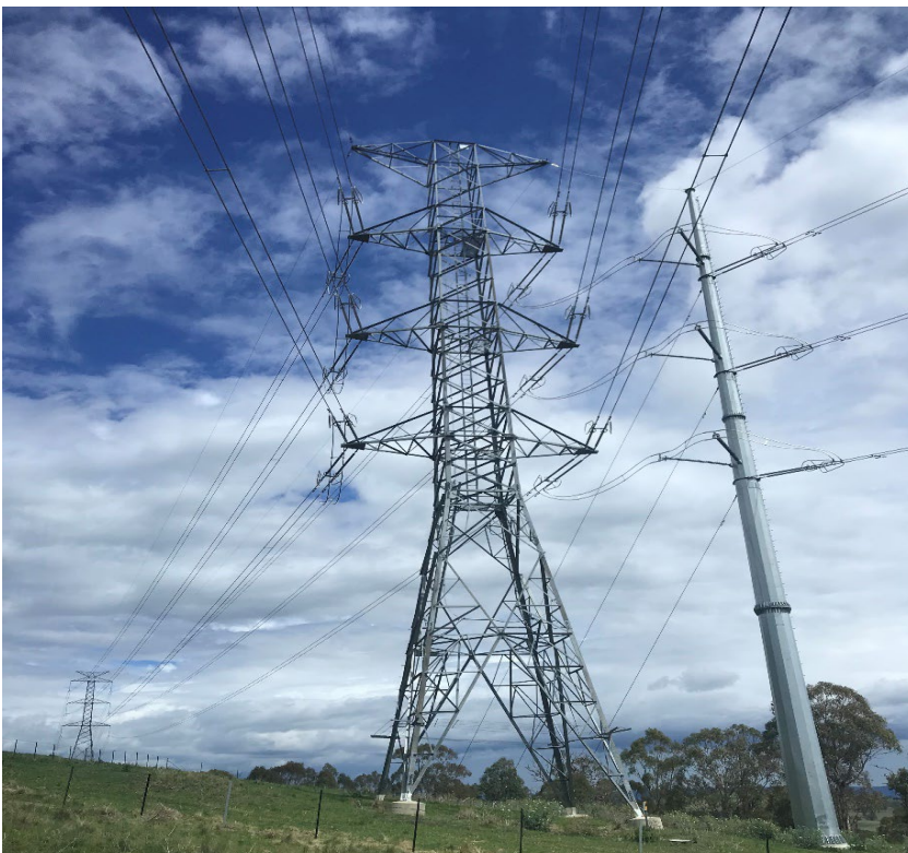
Figure 3.6 Example of double-circuit overhead 330 kV transmission line adjacent to a new single-pole substation tie-in
