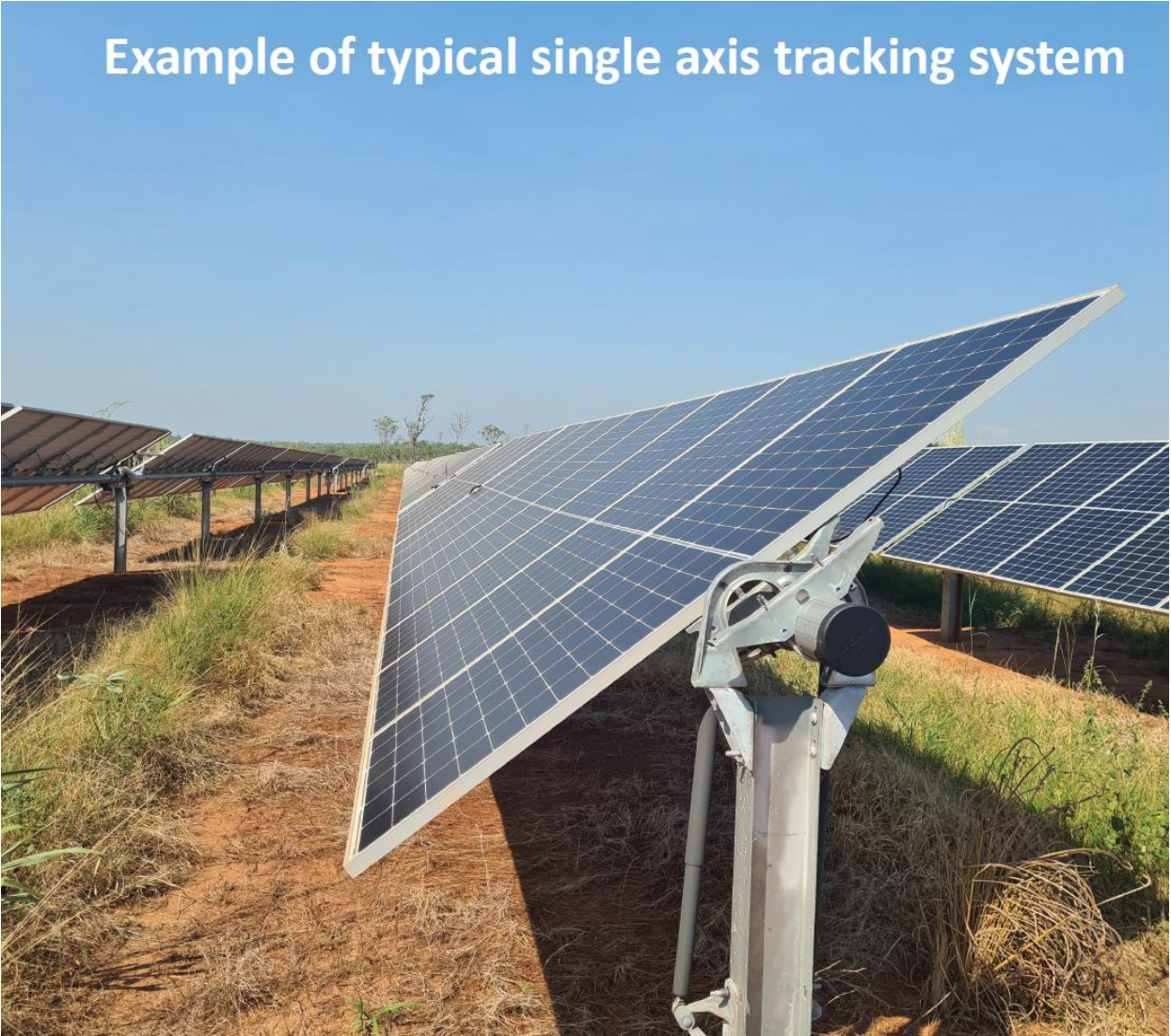
Figure 3: Example of single axis tracking system (approx. 0.8m high). System proposed at RVSF will be minimum of 2.5m above ground level at axis.
