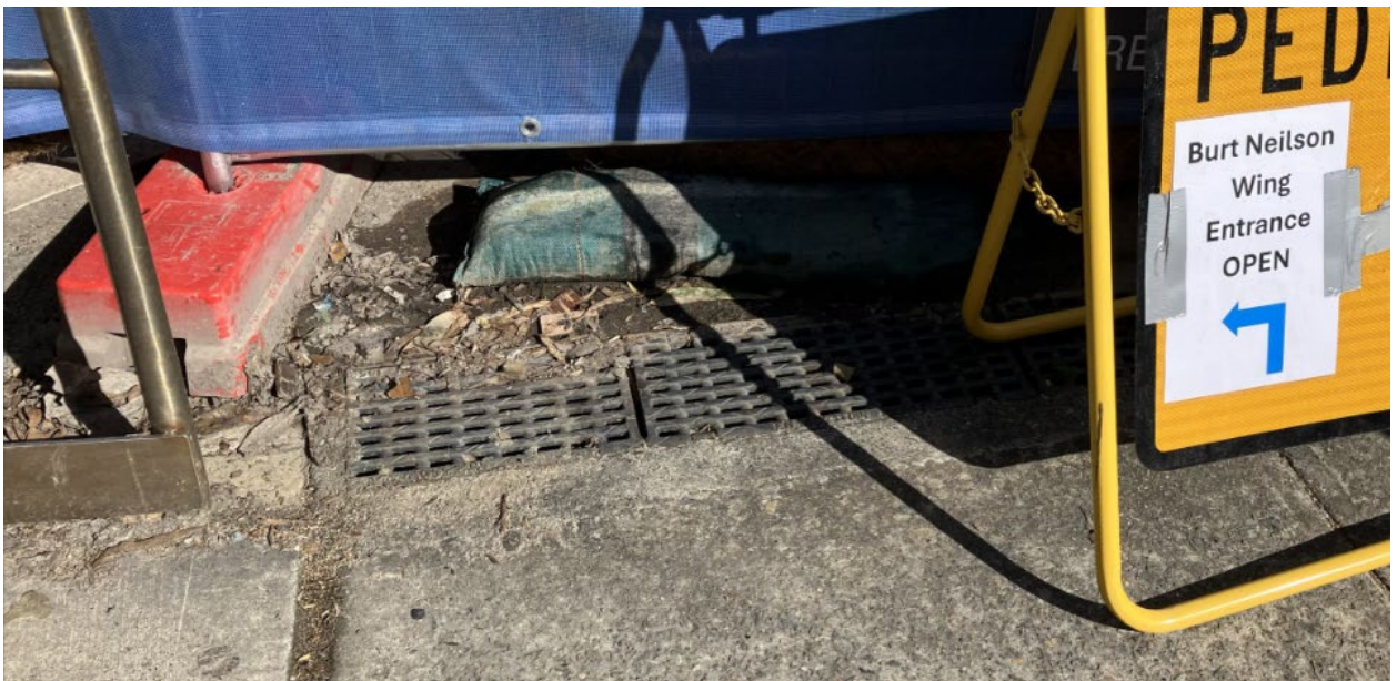
Site Observation OBS-01: Update to controls required at drainage pit at Kensington Street.
