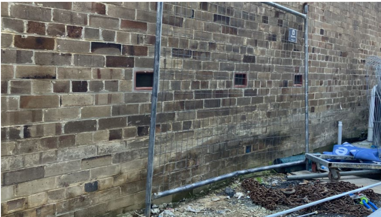
Site Observation OBS-02: Portion of fencing was observed to be leaning against the Heritage Wall.
