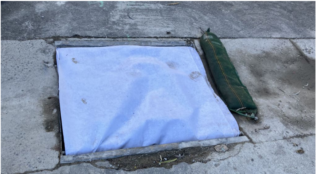
Site Observation OBS-01: Update to controls required at drainage pits at link bridge area as geofabric raised and can still let sediment in.
