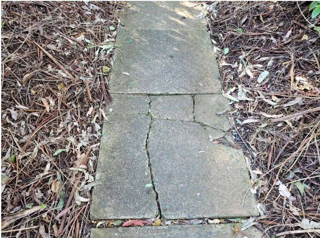
Photo 10: Cracks and Deformations present on footpath
