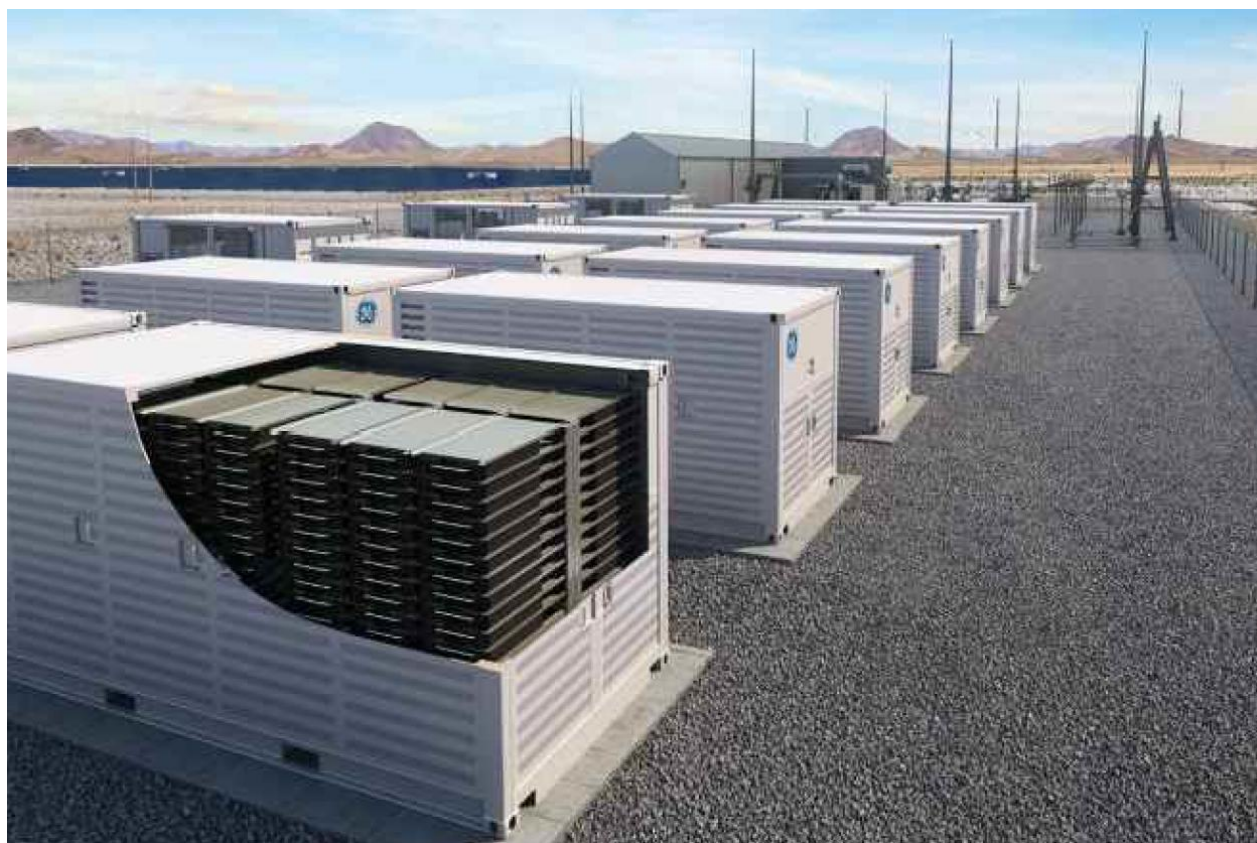
Figure 3-4: Typical BESS Arrangement
