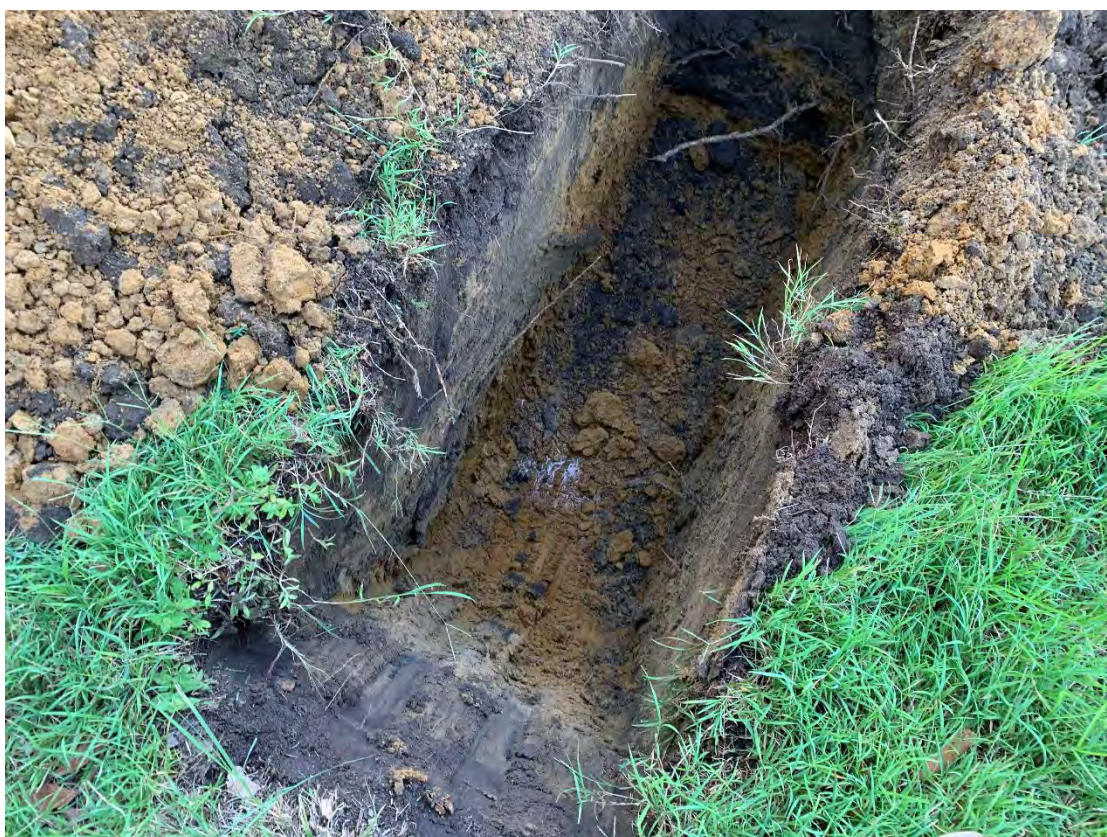
Photograph 16: Seepage observed in TP23
