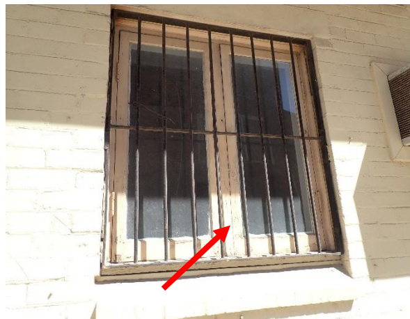
Photo 8: Residence – lead based brown/cream paint to the external timber windows
