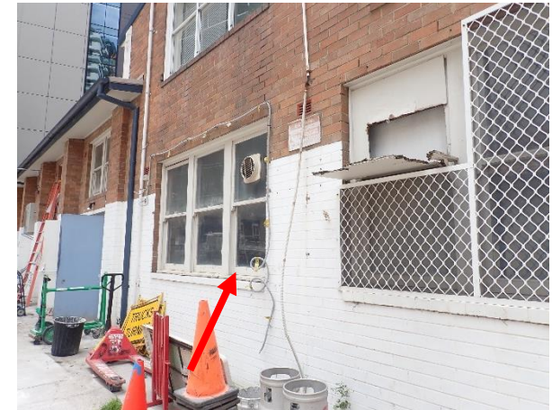
Photo 21: PCYC – lead based cream paint to the external timber windows
