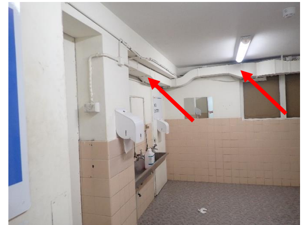
Photo 18: PCYC – assumed asbestos containing mastic to the air conditioning ducting within the south portion
