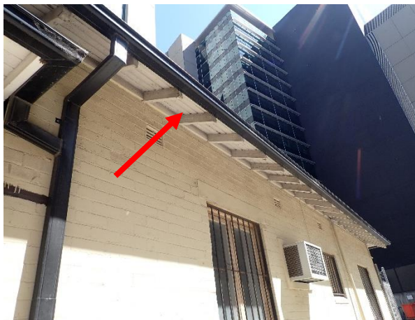
Photo 7: Residence – lead based white paint to the timber eaves & soffits
