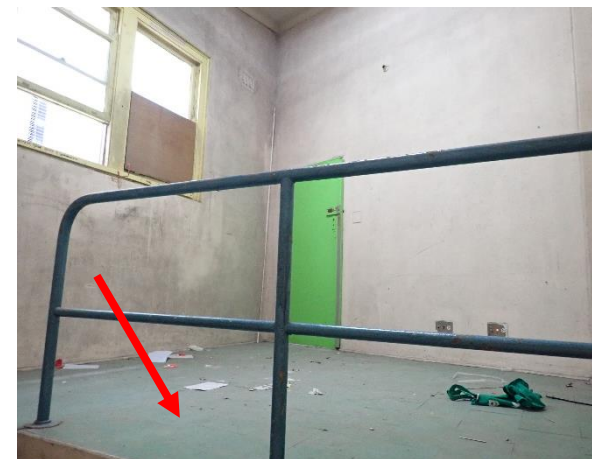
Photo 12: PCYC – asbestos containing green vinyl floor tiles to the northwest store room in the northwest portion
