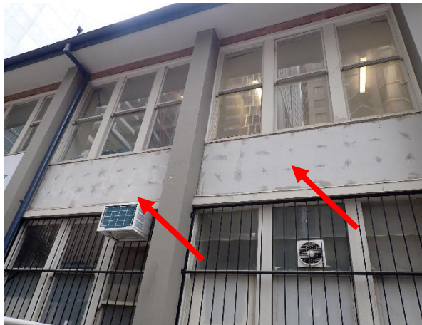
Photo 16: PCYC – assumed asbestos containing fibre cement sheeting to the south spandrel panels
