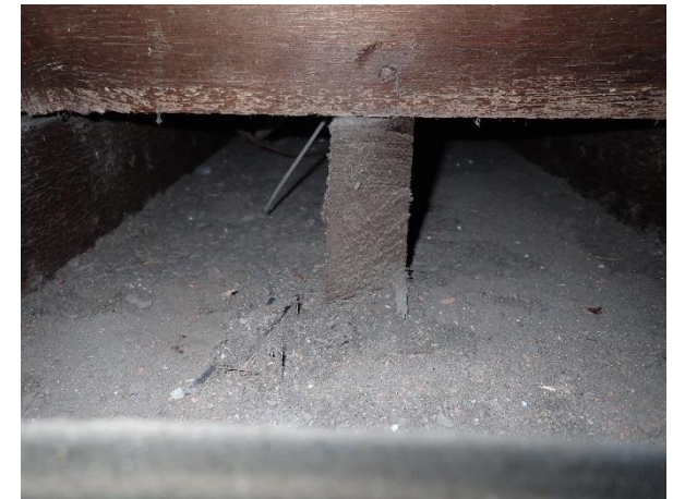
Photo 6: Residence – lead containing dust within the ceiling cavity
