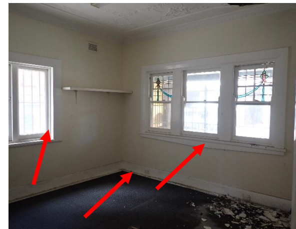
Photo 9: Residence – lead based white paint to the internal timber skirting boards, architraves and windows
