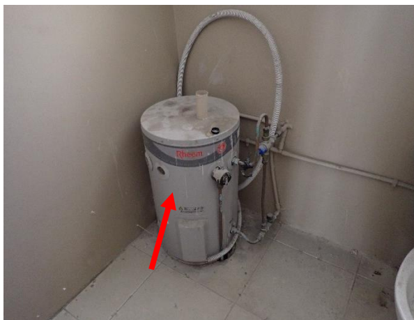
Photo 10: Residence – assumed internal SMF insulation to the hot water system in the bathroom
