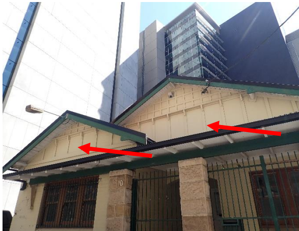
Photo 4: Residence – assumed asbestos containing fibre cement sheeting to the south gable panels
