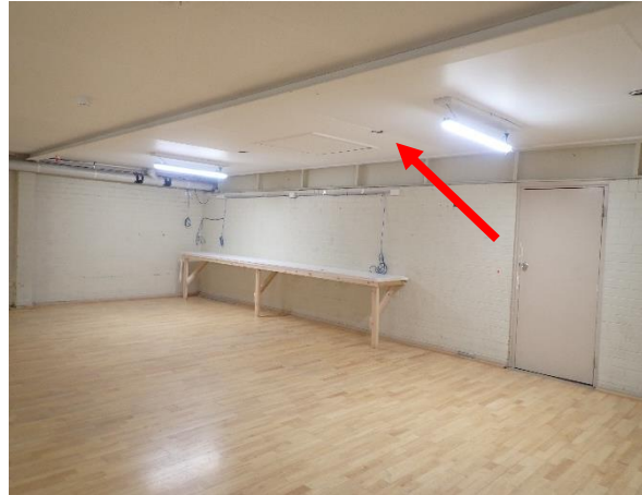
Photo 14: PCYC – asbestos containing fibre cement sheeting to the offices in the northeast portion
