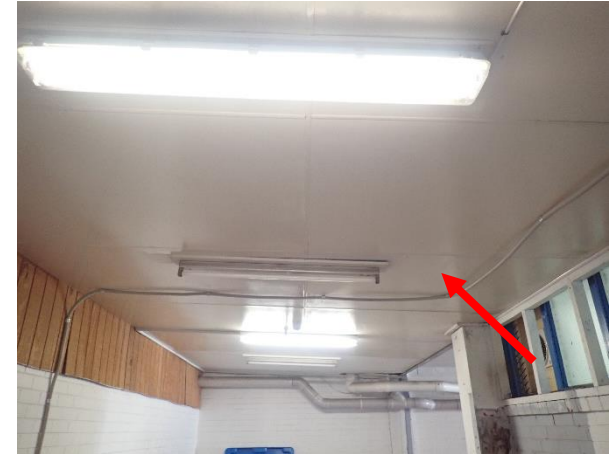
Photo 15: PCYC – asbestos containing fibre cement sheeting to the north ceiling of the garage
