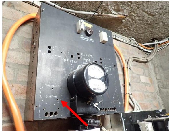
Photo 17: PCYC – assumed asbestos containing electrical backing boards within the south portion electrical room
