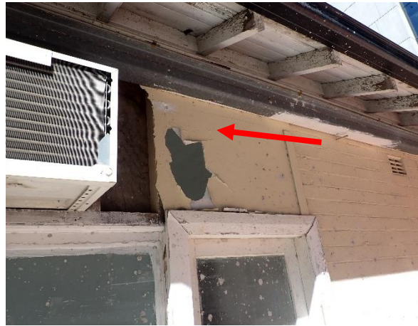
Photo 2: Residence – asbestos containing fibre cement infill panel above external kitchen door
