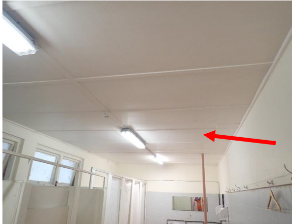
Photo 13: PCYC – asbestos containing fibre cement sheeting to the ceiling of the male toilets in the northeast portion
