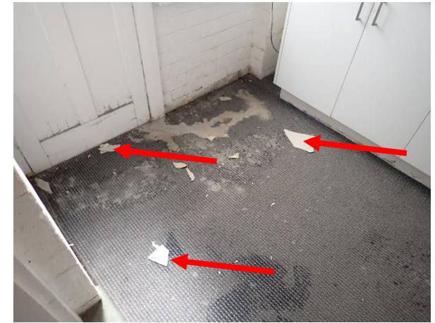
Photo 3: Residence – asbestos containing fibre cement debris on the floor of the kitchen
