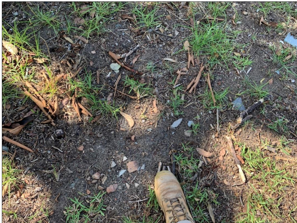
Photo 40: Demolition waste at the surface of former classrooms footprint including concrete, bricks, sandstone, pavers, PVC, agricultural pipe, PVC, metal and areas with multiple fibro fragments.
