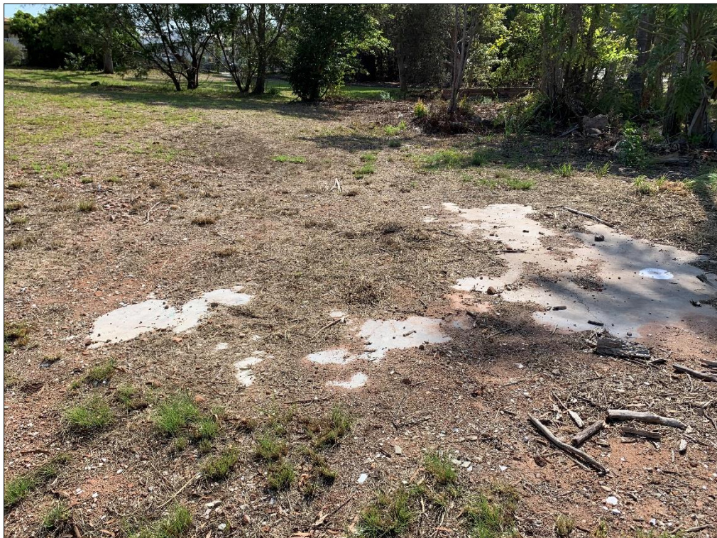
Photo 32: Scattered demolition waste and fibro sheeting within the to former administration building footprint.
