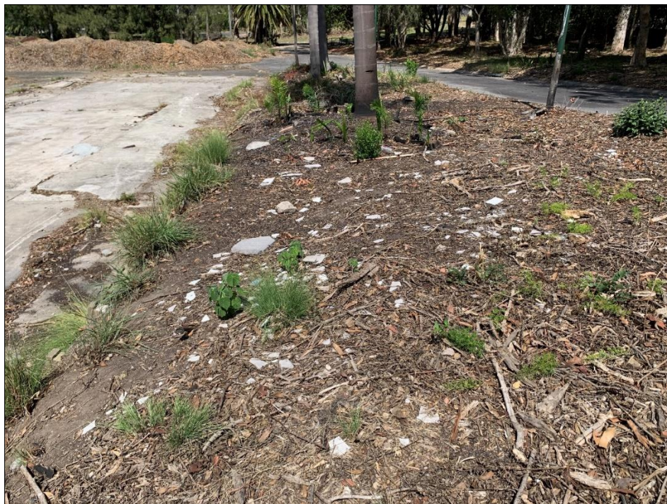
Photo 24: Garden bed south of the central hardstand area comprising abundant fibro sheeting fragments at the surface, looking east.
