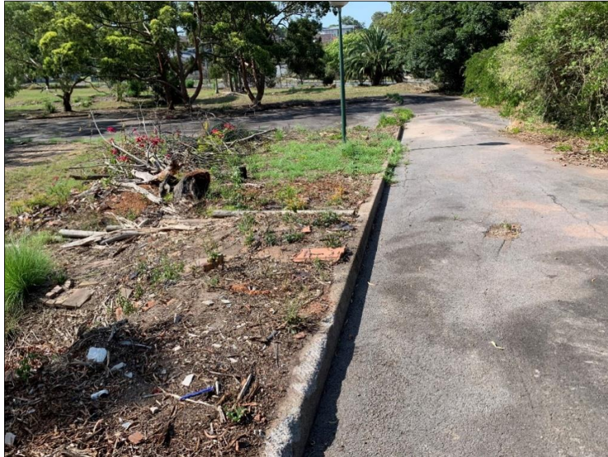
Photo 33: Scattered demolition waste and fibro sheeting adjacent to former administration building footprint, looking north.
