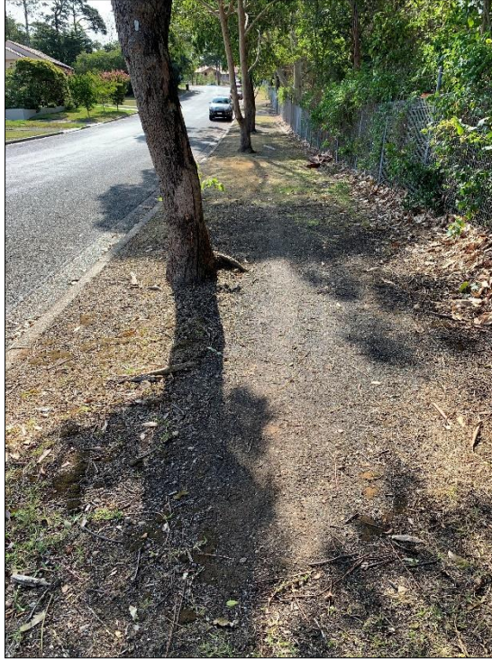
Photo 43: Possible black slag fill observed at the surface in the road shoulder near the drainage reserve road crossing on Tiral Street.
