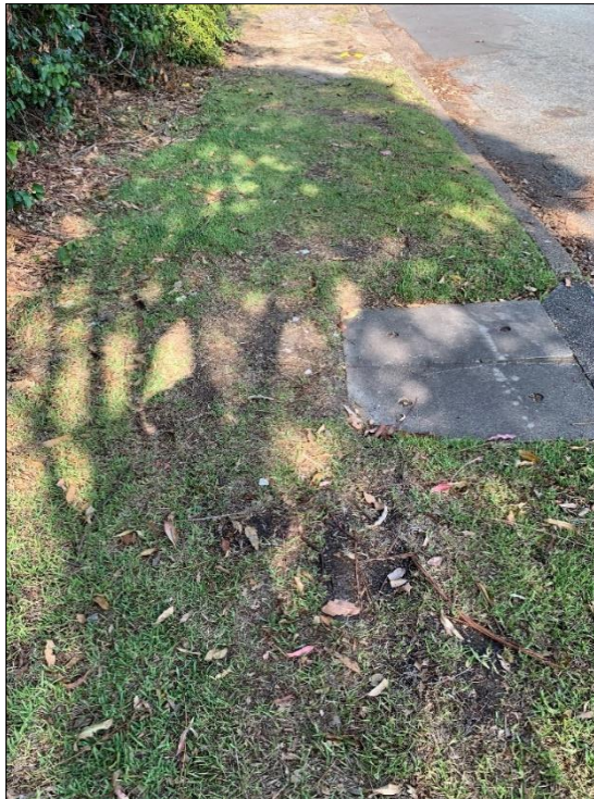
Photo 44: Fibro fragments observed on surface of road shoulder along Tiral Street.
