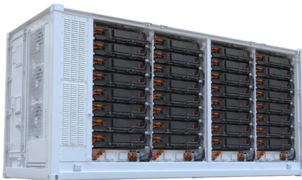
Figure 3-4: Typical Containerised BESS
