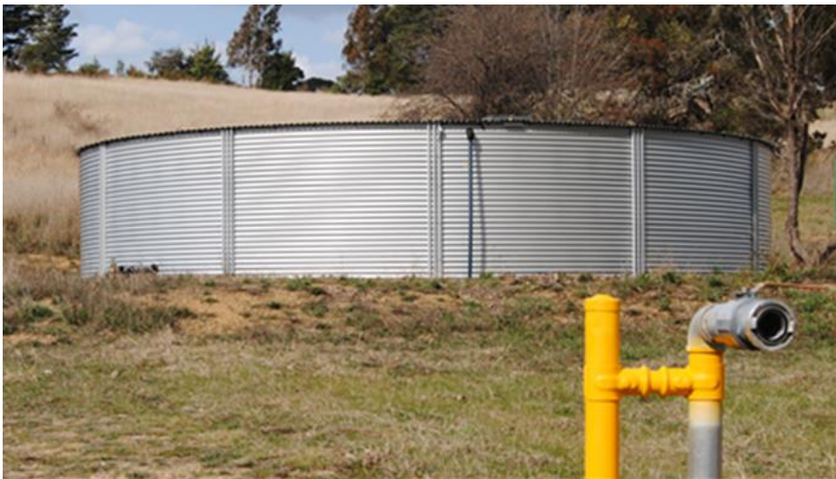
Figure 10 - Example of storz connection associated with a dedicated water storage tank used for dedicated firefighting purposes and a standard "Static Water Supply" sign to be placed at the front of the property.
