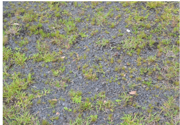
Figure 26. Patches of blue metal demonstrating imported fill.
