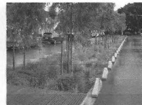
Car Park Centre Median Bioretention as landscape features to collect runoff and percolates through prescribed soil filtration media that is densely vegetated.
