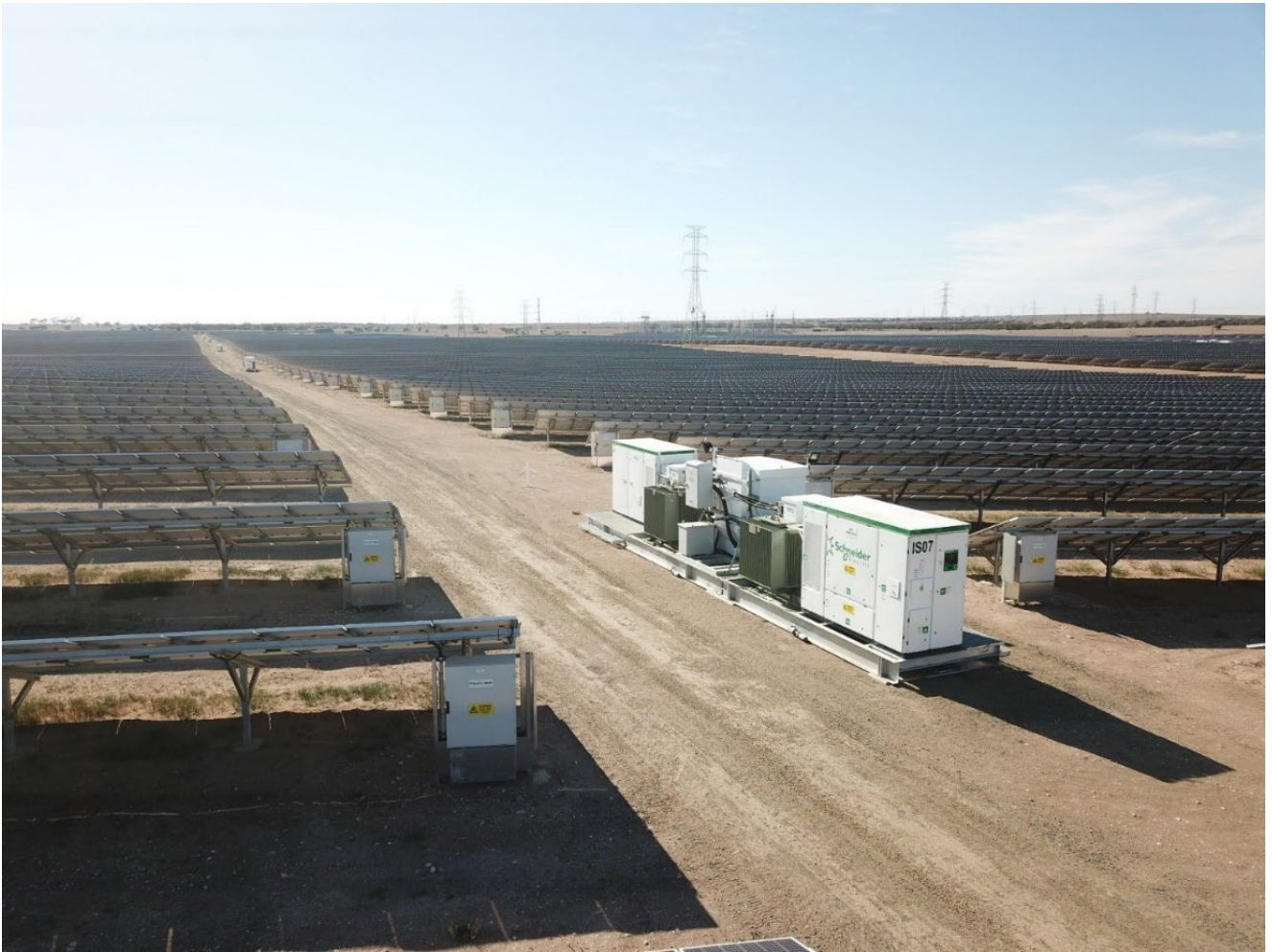
Photograph 3.2 Example of solar PV modules and inverter station at Tailem Bend, South Australia
