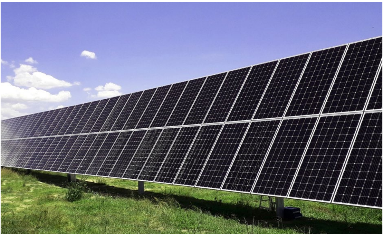
Photograph 3.1 Example of solar PV modules mounted to single axis tracking structures
