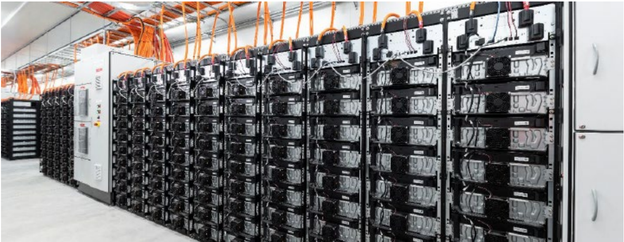
Photograph 3.3 Example of individual battery modules installed in racks and connected via cabling.
